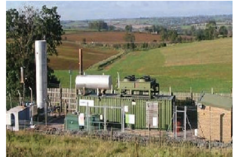
Figure 1.3 Landfill gas engine
