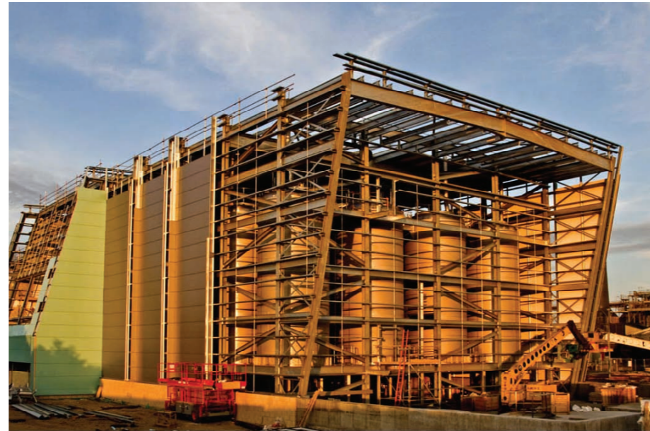
Figure 1.2 Roseisle distillery (which has an anaerobic digestion facility)
