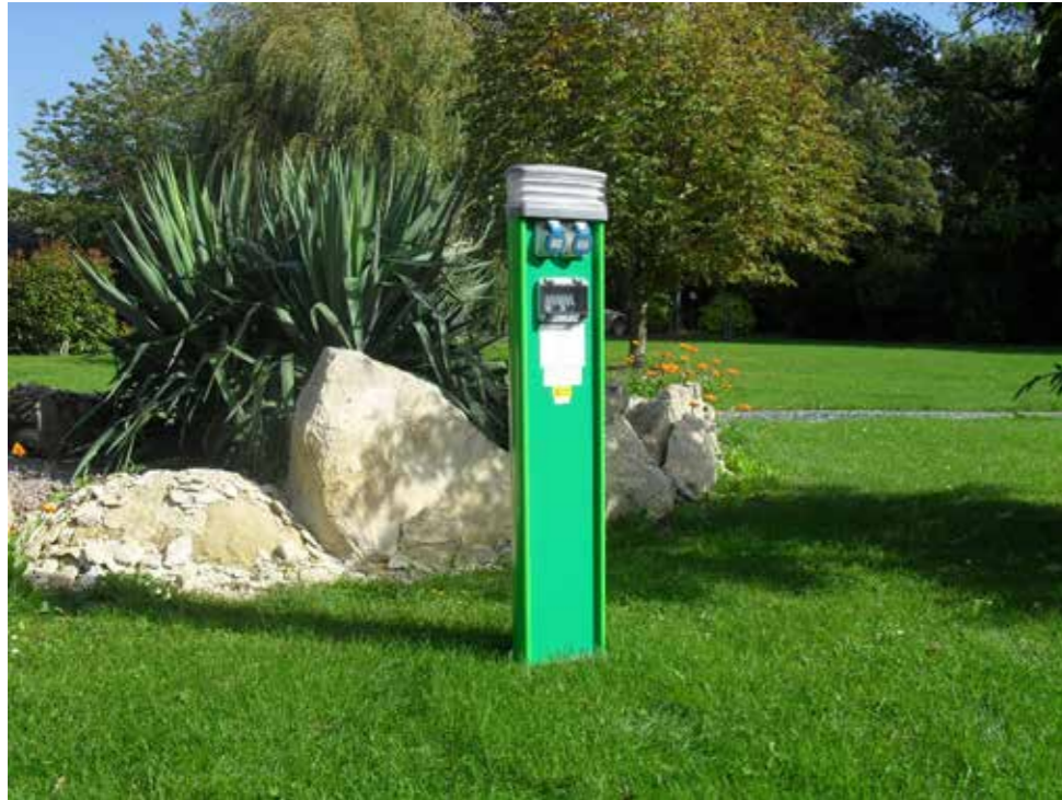
RMCS - Electrical Service Pedestal
