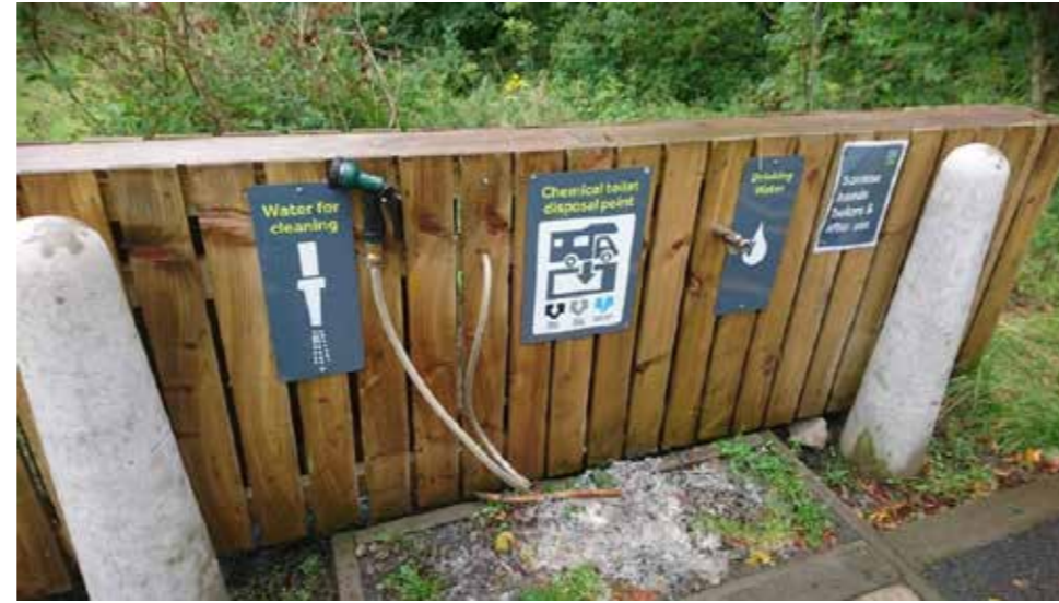
Example of new water supply with clear signage identifying wash down water, drinking water and chemical waste disposal point.
