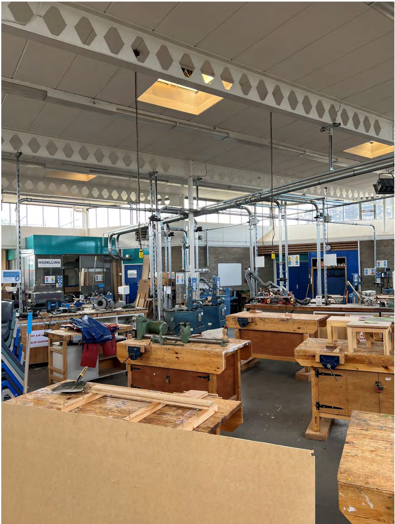
Photo N.13 Castellated beams supporting Siporex panels in Tech workshop – flange appears to be 165mm
