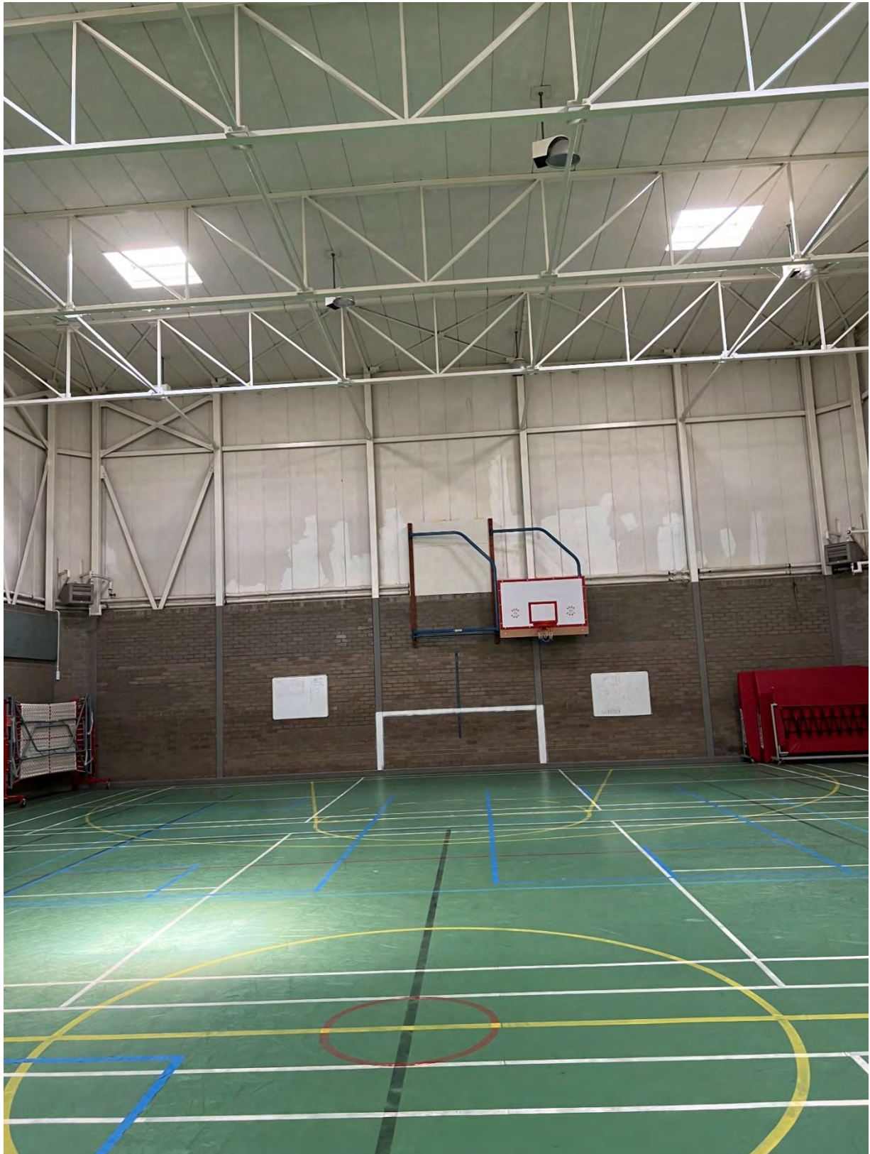
Photo N.11 Siporex roof panels supported on top chord of truss in gym area – bearing appears less than 75mm
