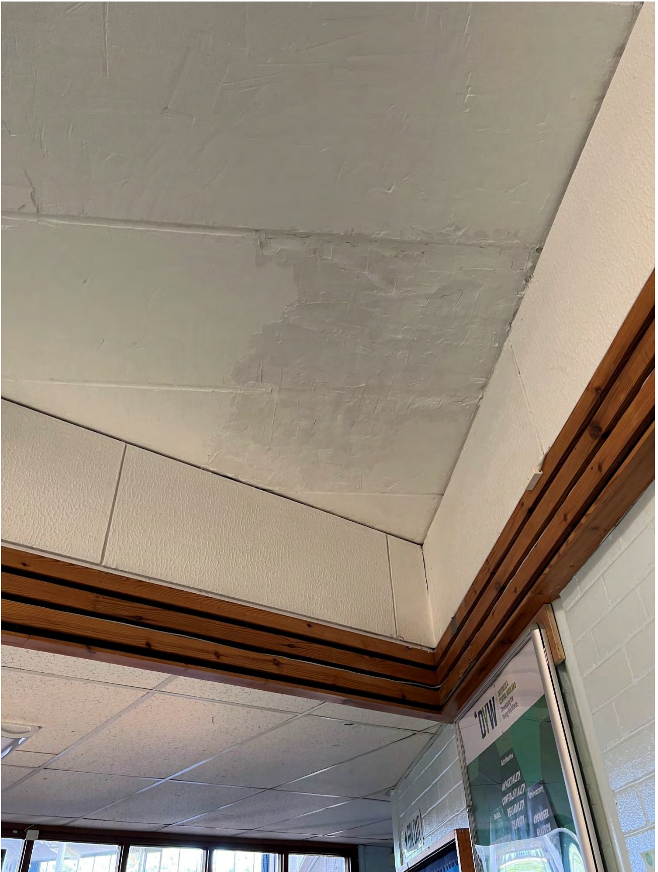
Photo N.3 Soffit of Siporex panels has been damaged during removal of asbestos coating
