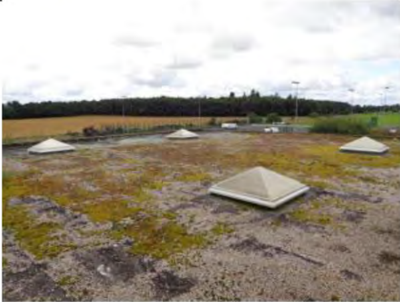
Photo No 7 – Games Hall Roof With Minor Organic Growth
