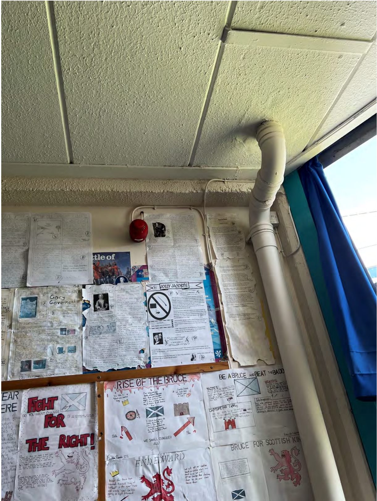
Photo N.5 pipework through panel is supported with correct bridle detail
