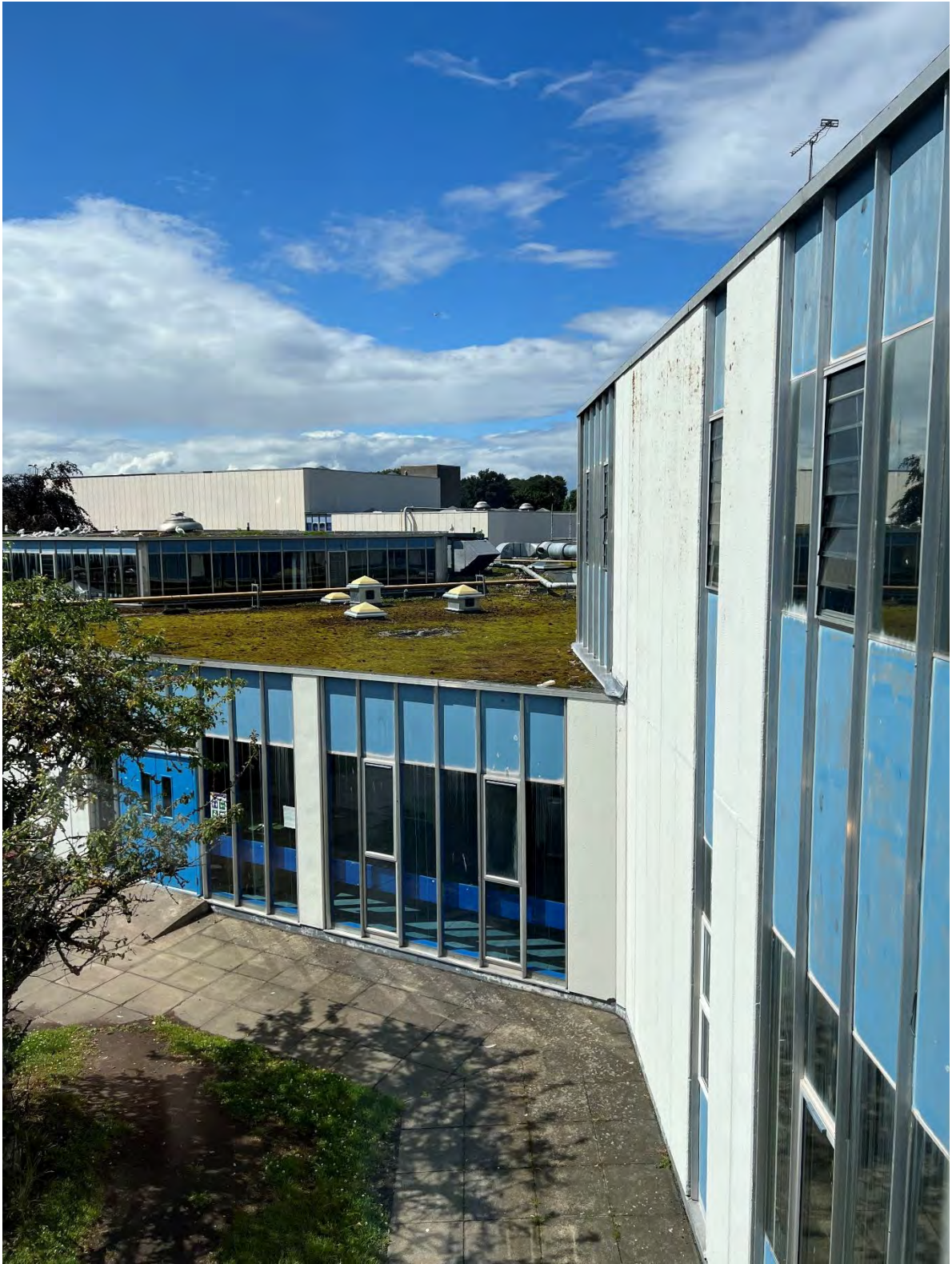
Photo N.8 Flat roofs externally have moss and vegetation throughout which will trap moisture
