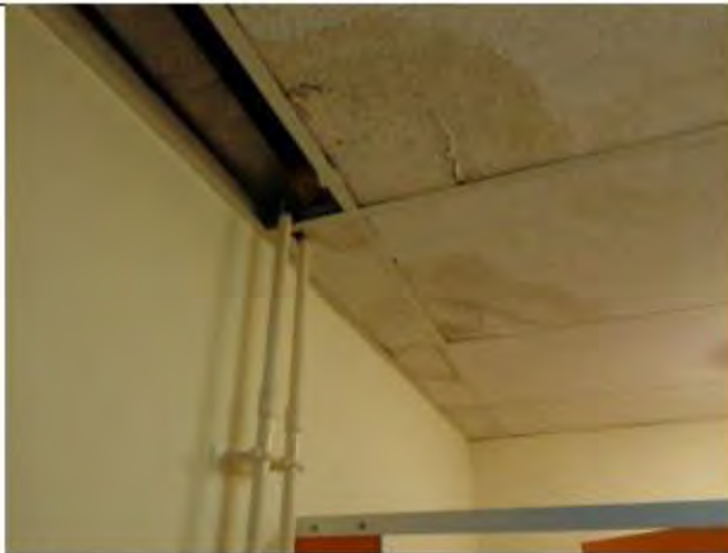
Photo No 10 – Historic Staining From Leaking Pipework
