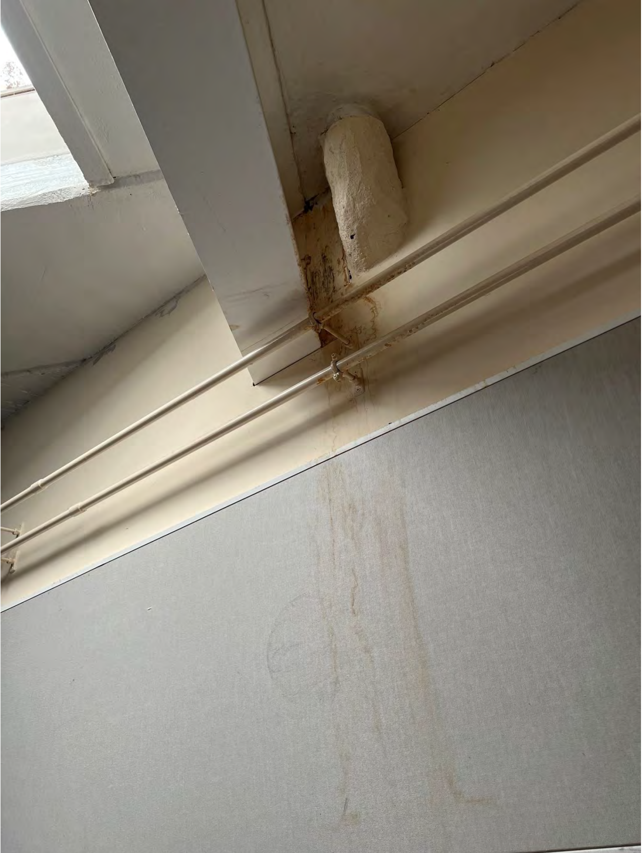
Photo N.12 water ingress at service pipe location no bridle to support slab penetration
