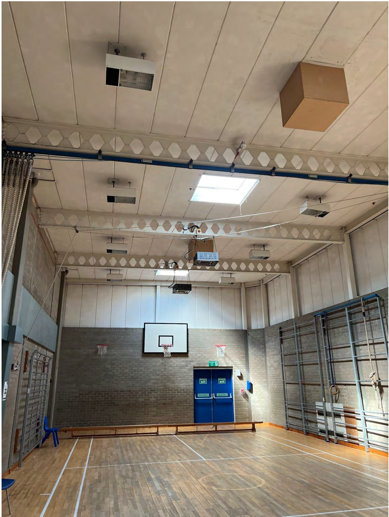
Photo N.10 Castellated beams supporting Siporex panels in gym – flange appears to be 165mm
