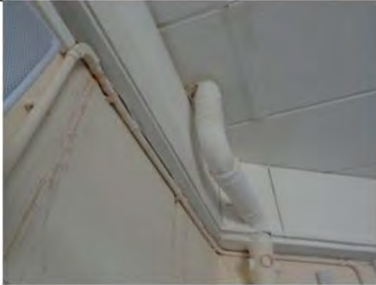
Photo No 11 – Earlier Repairs From Stormwater Drains & Water Pipes
