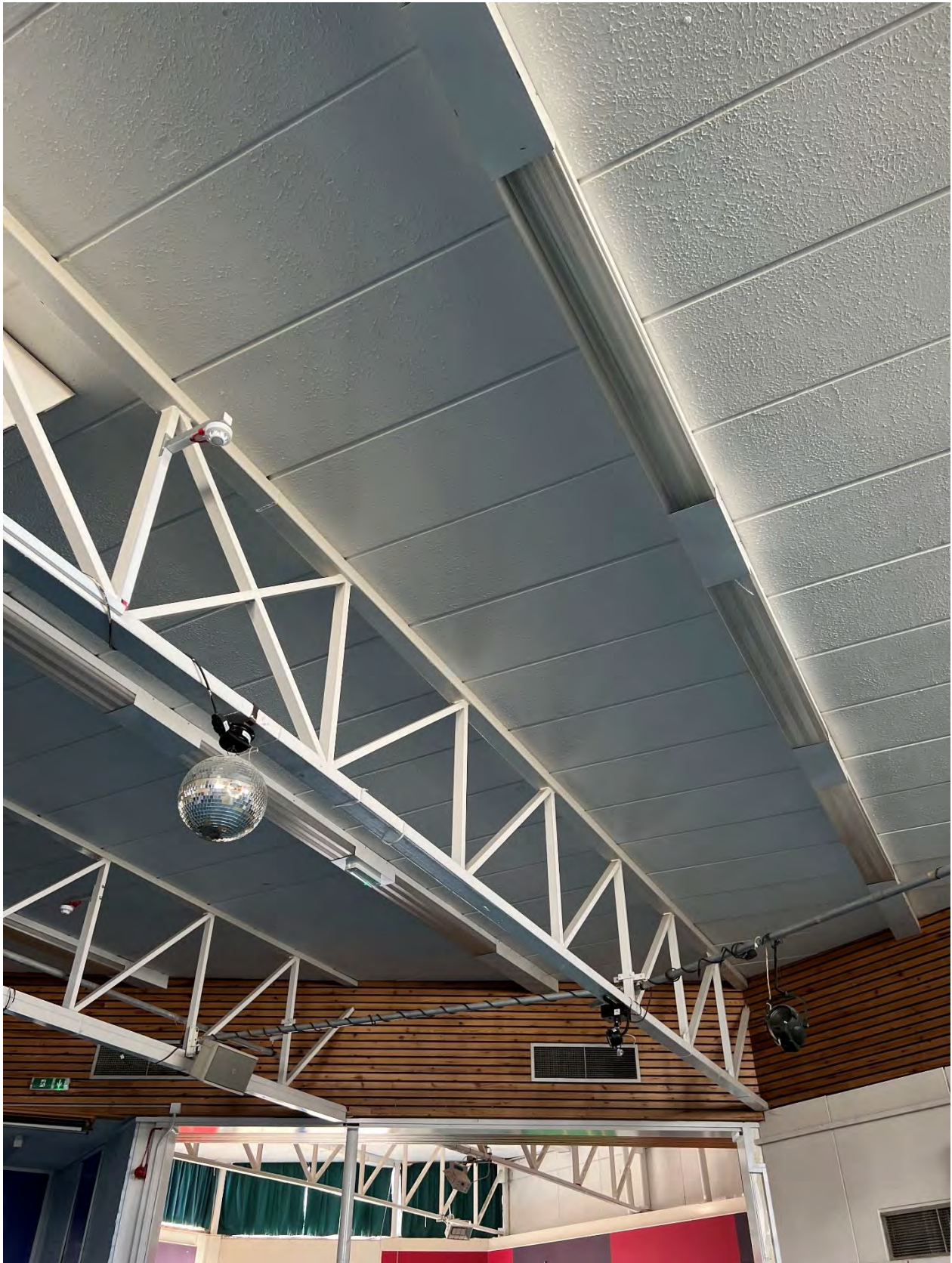
Photo N.9 Siporex roof panels supported on top chord of truss in canteen area – bearing appears less than 75mm
