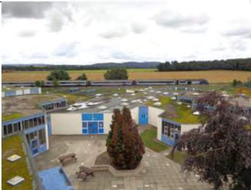
Photo No 6 – Roof Areas With Water Present
