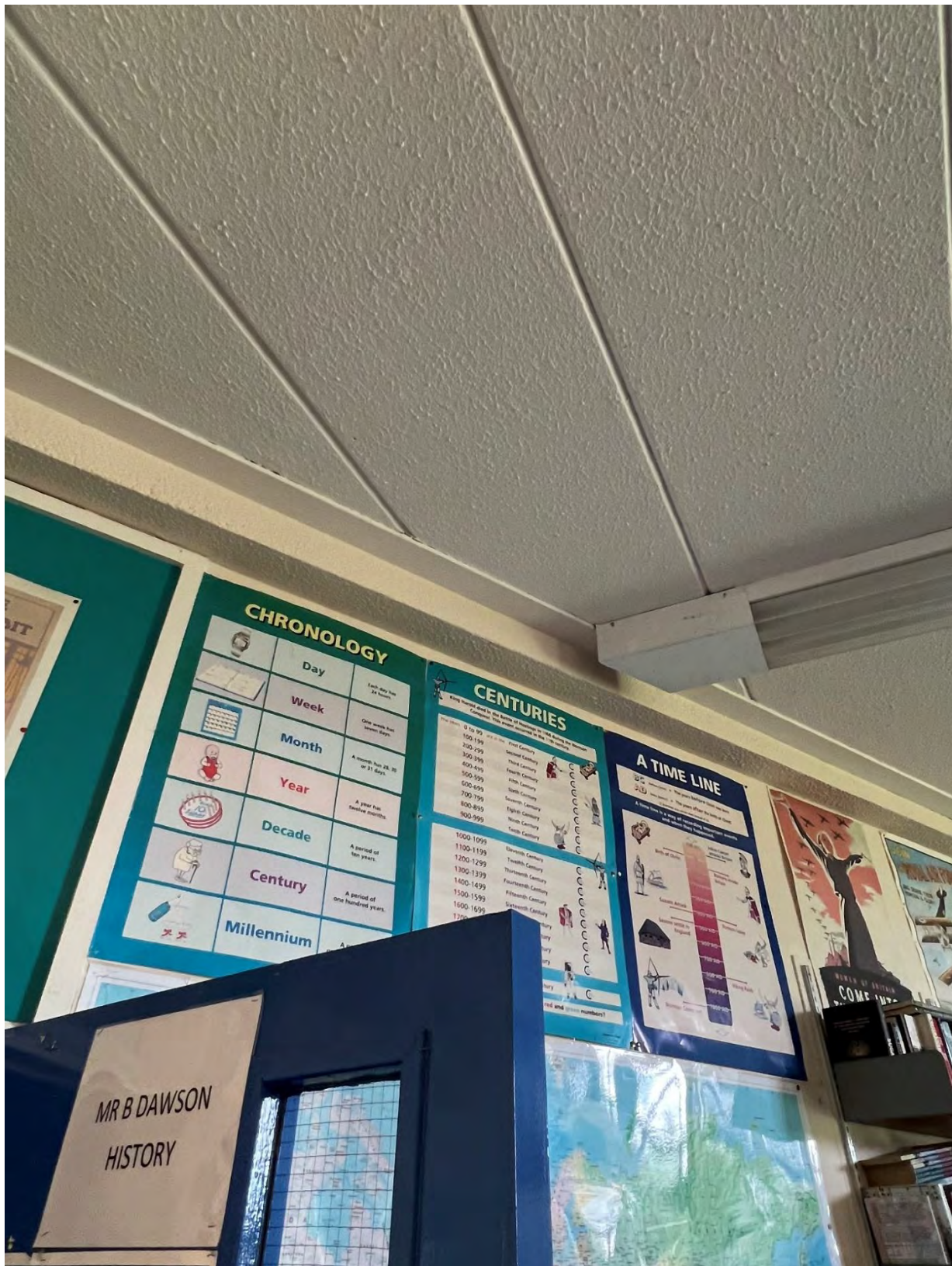
Photo N.6 Geometry of rooms mean the panels are not parallel to supporting beam – unclear on whether bearing length is more than 75mm across whole length
