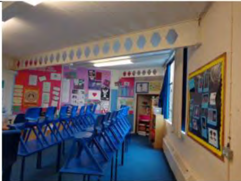
Photo No 12 – Some Panels Showing No Previous Damage Or Repairs
