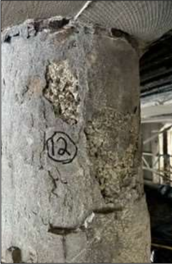
Identified Pile – repair determined.
