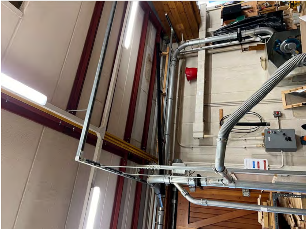
Photograph 8 – Technical Dept Workshop additional supports due to water ingress
