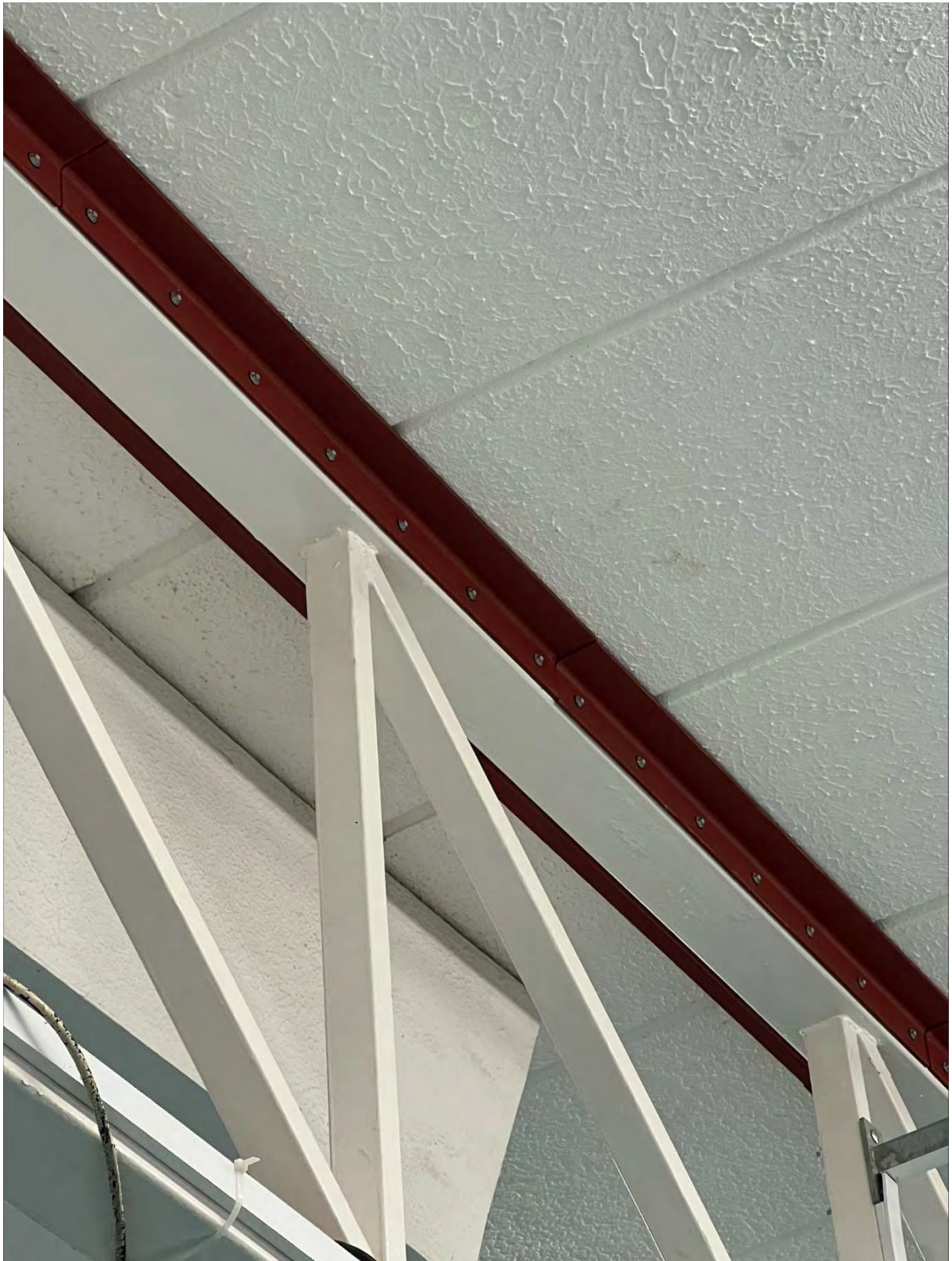
Photograph 7 – Dining Hall top chord bearing angle
