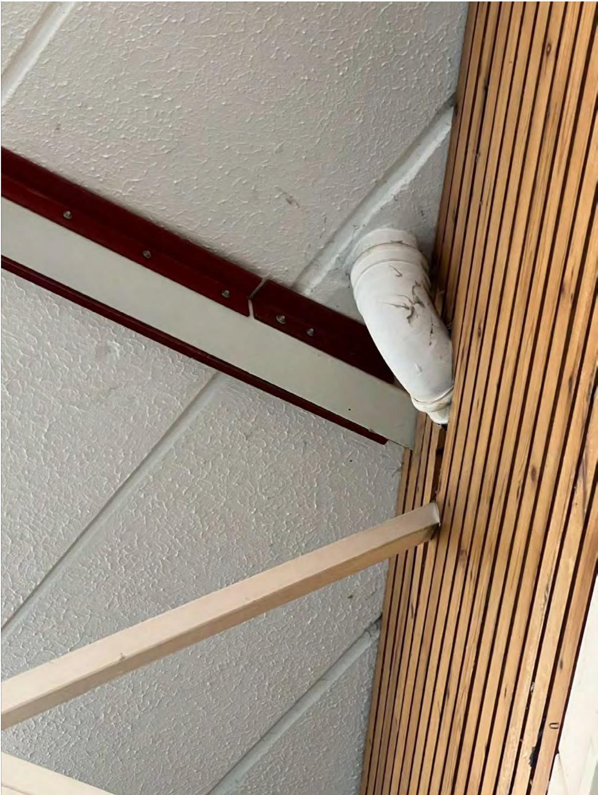
Photograph 8 – Dining Hall top chord bearing angle
