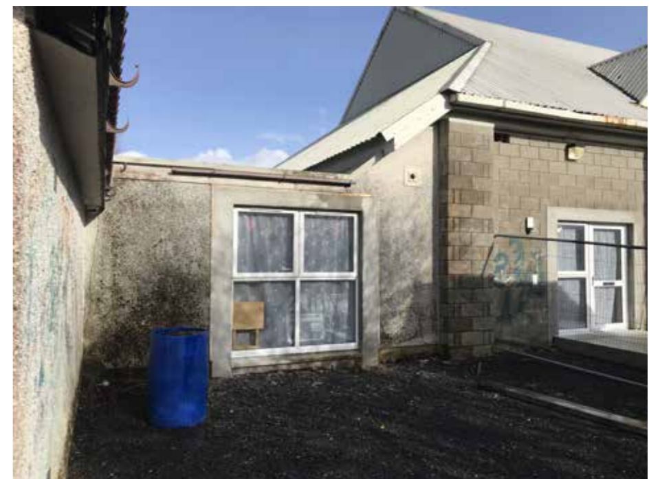
Rear of garage - note missing gutters
