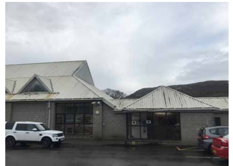
Entrance lobby - note damage to eaves
