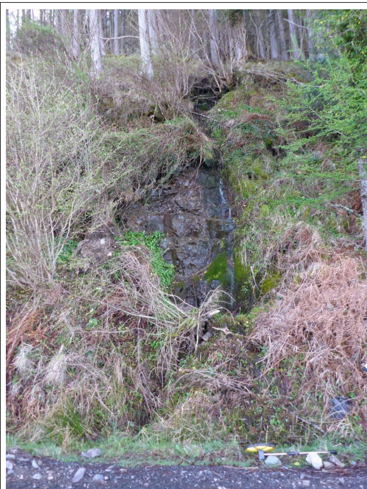
Photograph: AA2A-6 Ch. 476 – Small downslope watercourse over rockface. Vegetation and small blocks have been stripped and gathered at toe of slope. Year observation first noted: 2024
