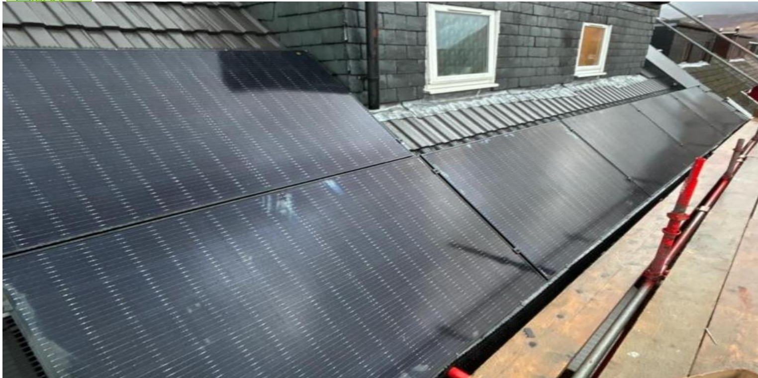
Figure 3 – PV panels on property
