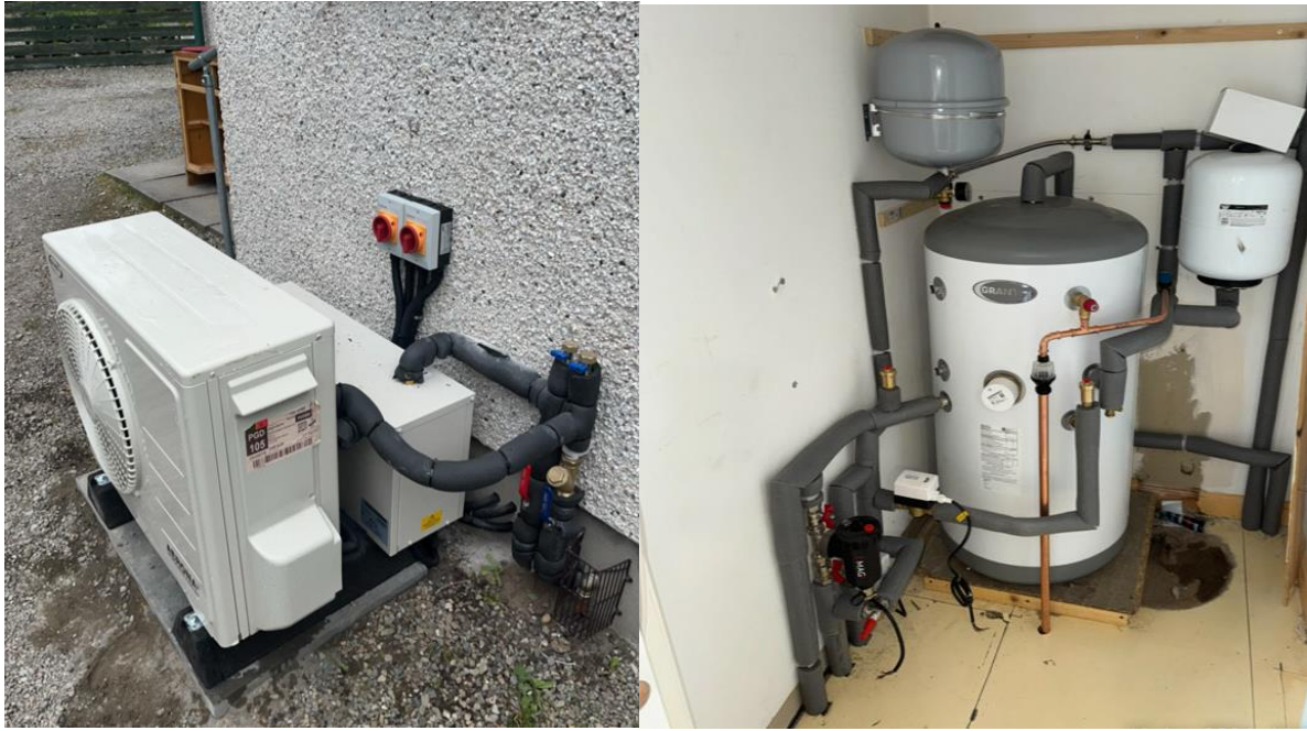
Figure 1 – ASHP and tank
