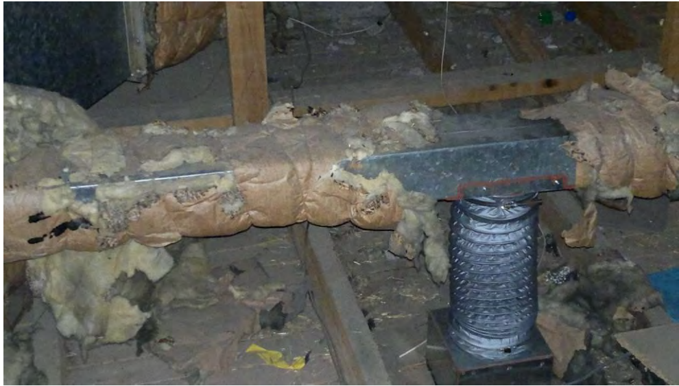
Figure 2 Supply duct and ceiling
