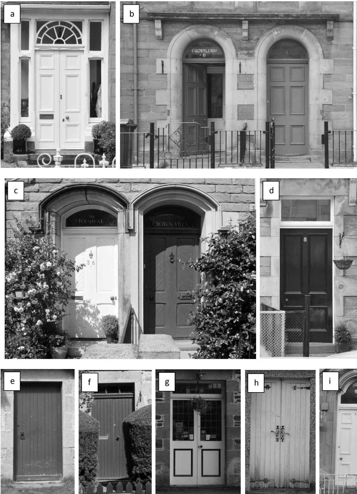
a: Double-leaf or bivalve 6-panel door with decorative fanlight and side lights; b: Pair of single-leaf 6-panel doors; c: Pair of 4-panel doors with decorated panels and detailed moulding; d: Refined 4-panel door with full-pane fanlight, note original handle, bell and keyhole; e: single-leaf plank and batten door; f: double-leaf plank and batten door with top light; g: pair of traditional half-glazed or casement doors; h: plank and batten door with attractive cast iron door furniture; i: double margin door.
