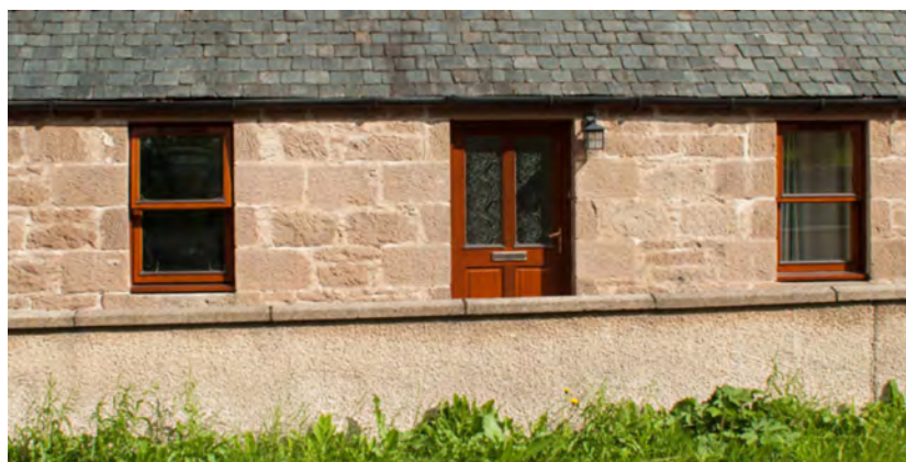
Timber effect uPVC door with glazed panels which detracts from the character and appearance of the traditional cottage.
