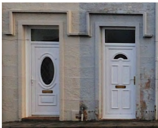
Standard white uPVC doors; never acceptable in a conservation area.
