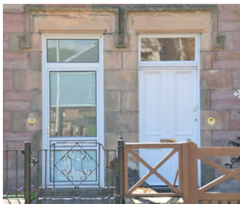
A half glazed inappropriate modern aluminium door, the poor finish, appearance and style accentuated by the adjacent traditional timber 4 panel double margin door.
