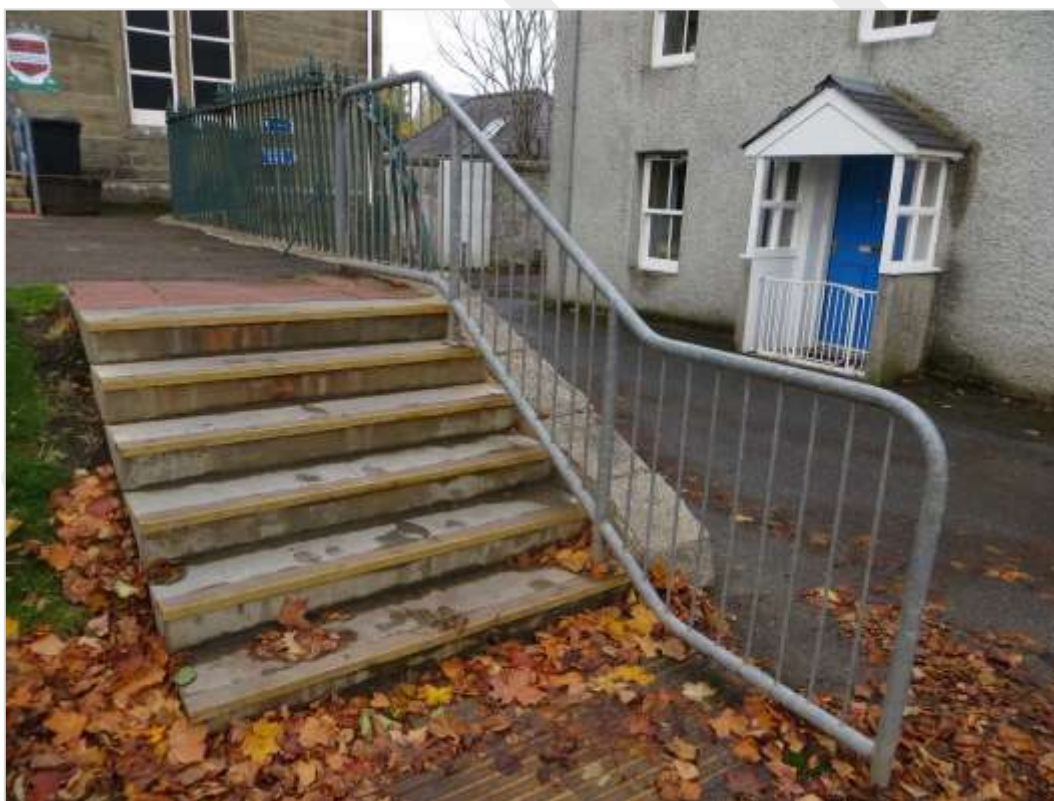
Fig 36: The steps adjacent to the former Court House are utilitarian and their appearance detrimental
