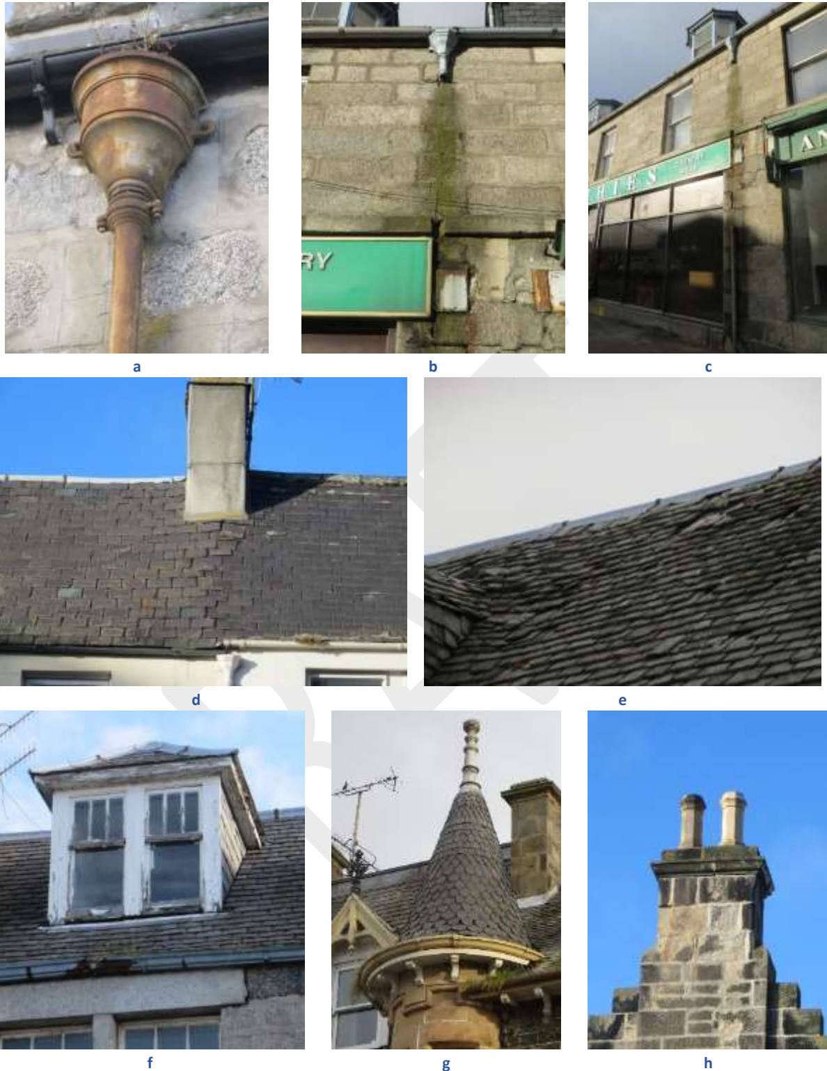
Fig 31 : Examples of disrepair: cast iron in need of painting and missing rainwater goods (a-c); slates poorly laid at the junction of 2 properties - possibly original cope stones have been removed (d); missing slates (e); timber dormer in need of repainting (f); blocked gutters (g); and eroded high level stonework (h).
