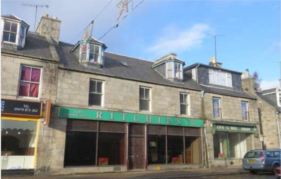
Fig 34: Vacant retail units and upper floors on High Street with repair issues.
