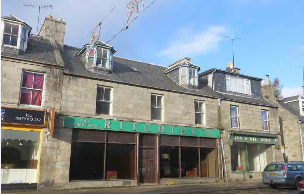
Fig 34: Vacant retail units and upper floors on High Street with repair issues.
