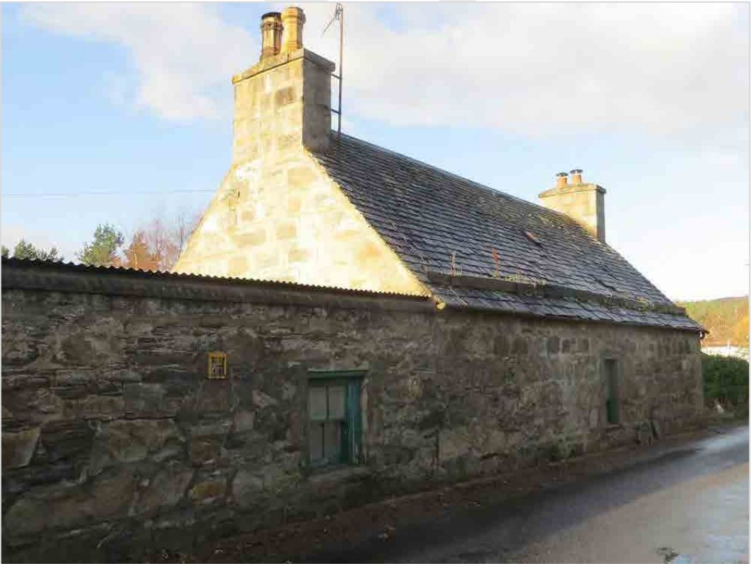
Fig 35: Vacant early cottage and boundary walls on Dunstaffnage Brae outwith the conservation area.
