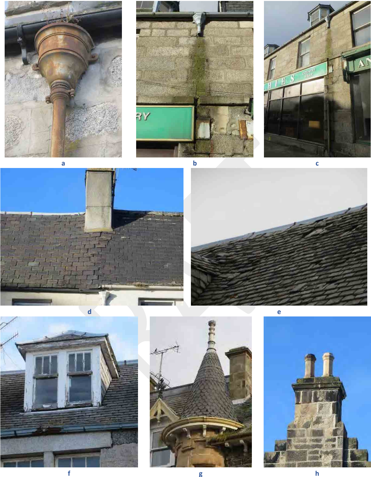
Fig 31 : Examples of disrepair: cast iron in need of painting and missing rainwater goods (a-c); slates poorly laid at the junction of 2 properties - possibly original cope stones have been removed (d); missing slates (e); timber dormer in need of repainting (f); blocked gutters (g); and eroded high level stonework (h).
