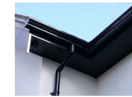
2 - Black PVC Drain Pipes
