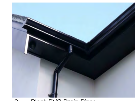
2 - Black PVC Drain Pipes
