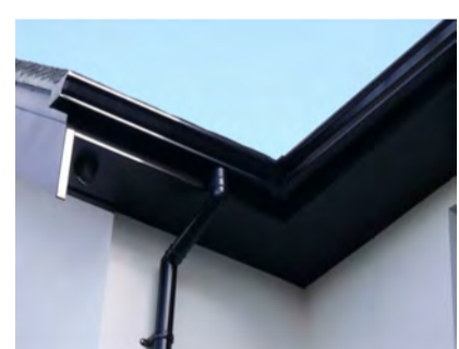
2 - Black PVC Drain Pipes
