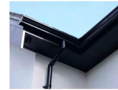
2 - Black PVC Drain Pipes
