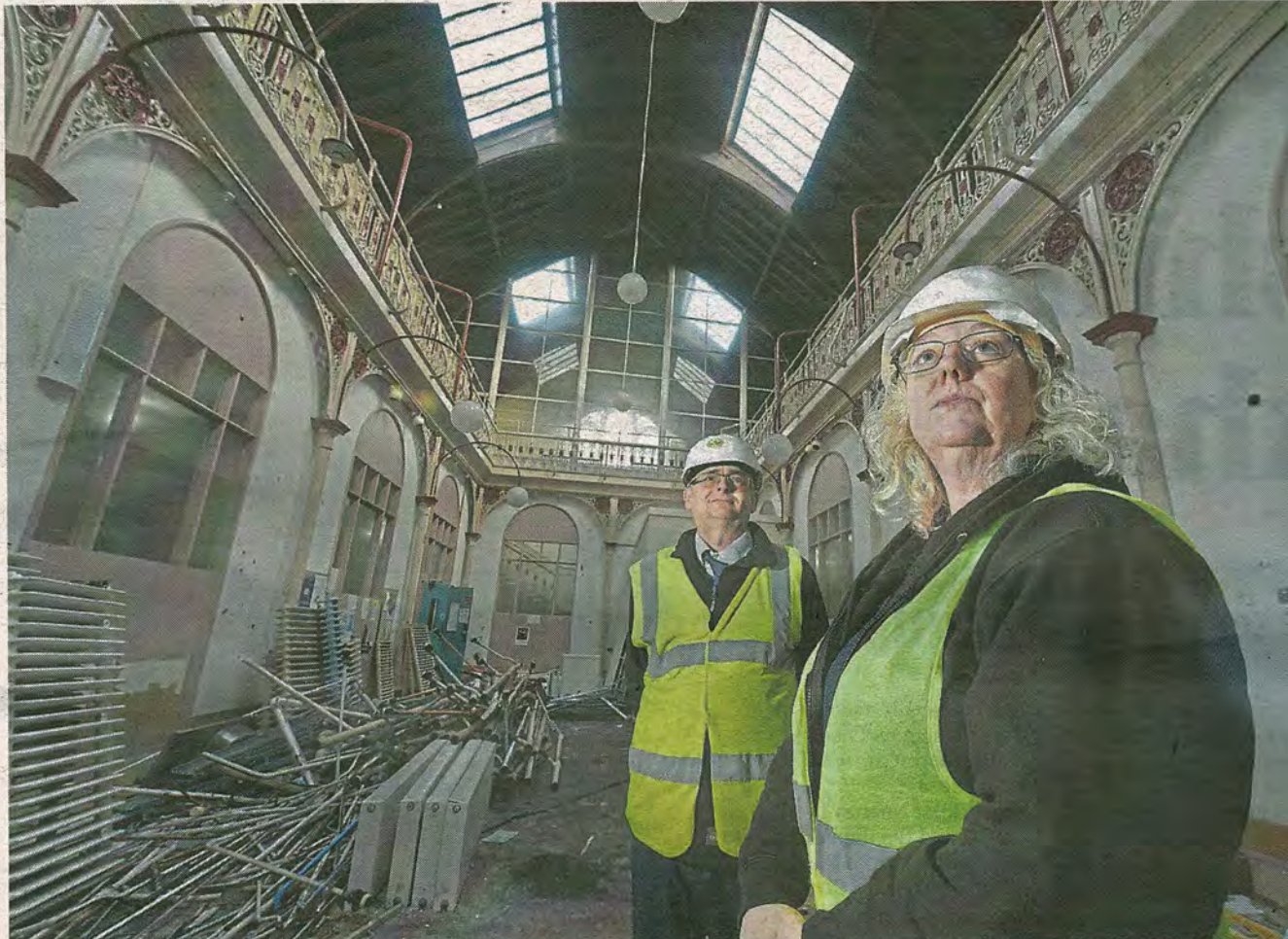
PROGRESS: Property manager Catherine MacNeil and Steven Leith of contractors Bancon at the old academy. Photograph by Sandy McCook
