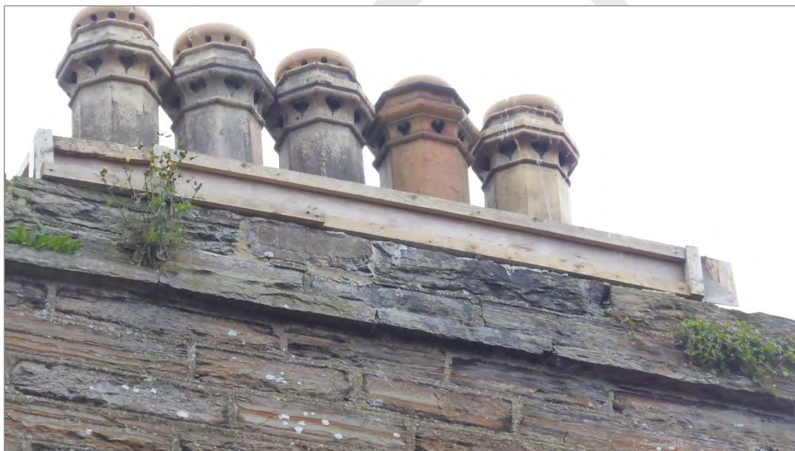
Figure 33: a typical Pulteneytown chimney with a thin flagstone slab forming a projecting tabling course detail before a further one or two courses of stone form the cope. Here with more elaborate hexagonal buff coloured chimney pots.
