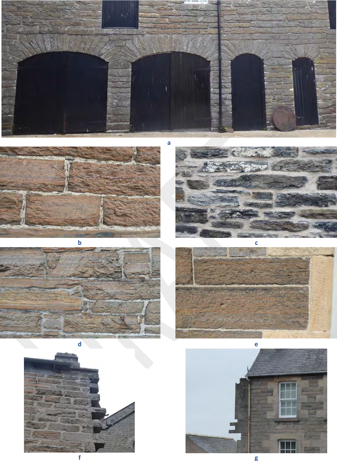
Figure 29: Masonry details: a: very fine examples of the segmental arches used in Pulteneytown particularly in the industrial buildings and to access internal yards, here at the Wick Heritage Centre; b: squared blocks of a warm brown Caithness stone with lime mortar and slate pinnings; c: walling recently repointed in lime on Saltoun Street warehouse, note the stones are more irregular in shape and darker grey in colour; d: a similar wall on a domestic property with irregular stones and courses, the gaps made up in smaller stacked stones; e: shaped Caithness stones on a Victorian building, cut to size, and used with sandstone dressings for openings; f and g: examples of masonry with projecting stones, known as ‘tusking stones’ or ‘tuskers’; left for bonding into the adjoining façade; image g showing the dressed window stones for the next property.
