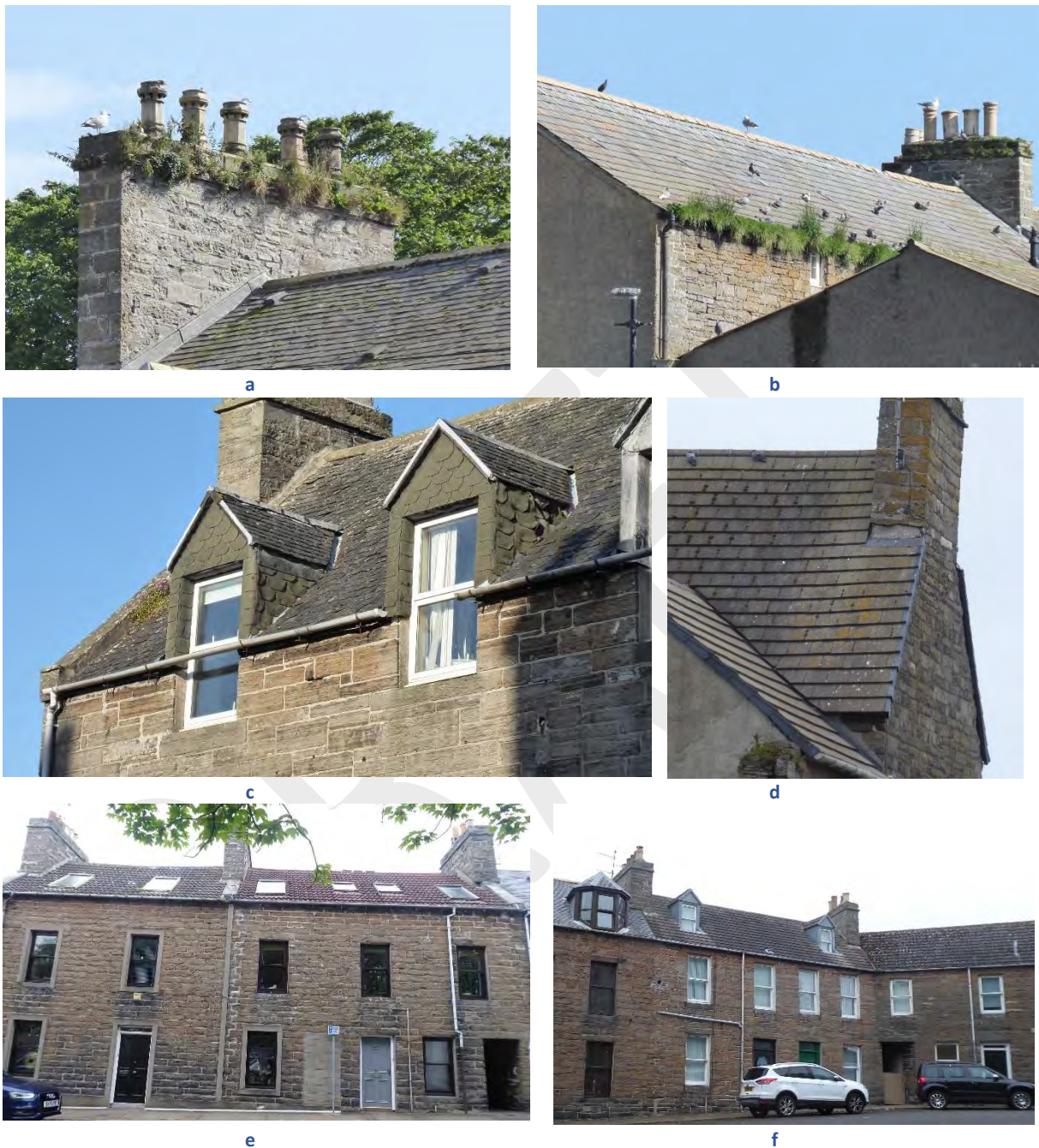
Figure 36: two common examples of vegetation growth leading to different defects and courses of action: a: plants taken root in open mortar joints in the masonry chimney. This is significant and roots unattended will continue to grow into the masonry and expand, over time destabilising the chimney stack; b: grass growing in a presumably blocked gutter with debris forming a soil for the vegetation. Here the blockage will lead to dysfunction of the rainwater system and overflowing of rainwater over the masonry walls and potentially backing up under the roof slate into the interior of the building; c: inappropriate materials, felt tiles, applied to two traditional gabled dormers; d: concrete tile replacement roof with possible removal of stone copes at the gable wall head, replaced by a plastic edge trim; e & f: inappropriate tile roof replacements on the terraced rows in Argyle Square; e: two different tiles, one red in colour both with large replacement rooflights; f: again two different tile finishes with a new slate finish on the left and a later large canted bay dormer.
