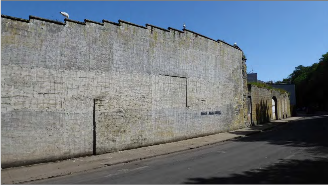
Figure 10: high masonry wall enclosing a plot on Union Street has a negative impact in terms of scale, materials, quality and monolithic style. It is unclear if original masonry fabric may survive below the rendered finish; earlier buildings on this site can be seen in historic images (e.g. fig 8)
