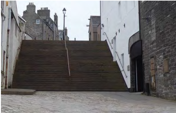
Repair of Black Stairs and streetscape enhancement using Caithness flagstones; part of THI 2008
