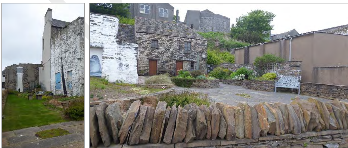
Figure 8: the Memorial Garden opposite the former boat yard site; on the left 3-storey walls of a former building have been consolidated and painted white, paint finish is failing.
