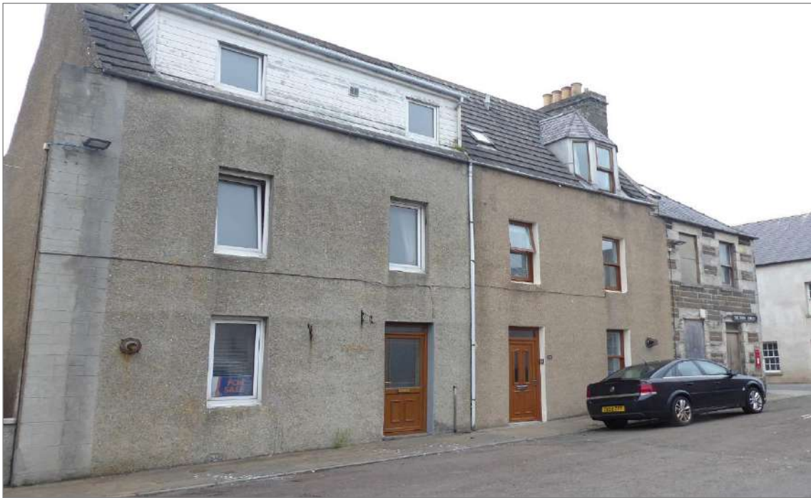
Figure 10: Inappropriate alterations: an example of past unsuitable change to a traditional building of heritage value which results in a negative impact. The original Caithness stone has been covered by a modern cement finish, the original windows and doors have been replaced; the window design and opening method has been altered; a large box dormer has been constructed which changes the form of the roof and obscures the original pitched slope; the original slate finish has been replaced in concrete tile. Buildings such as this can be enhanced and restored when opportunities arise through planning management.
