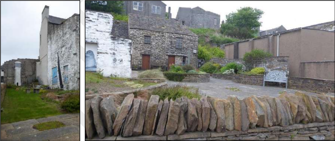
Figure 8: the Memorial Garden opposite the former boat yard site; on the left 3-storey walls of a former building have been consolidated and painted white, paint finish is failing.
