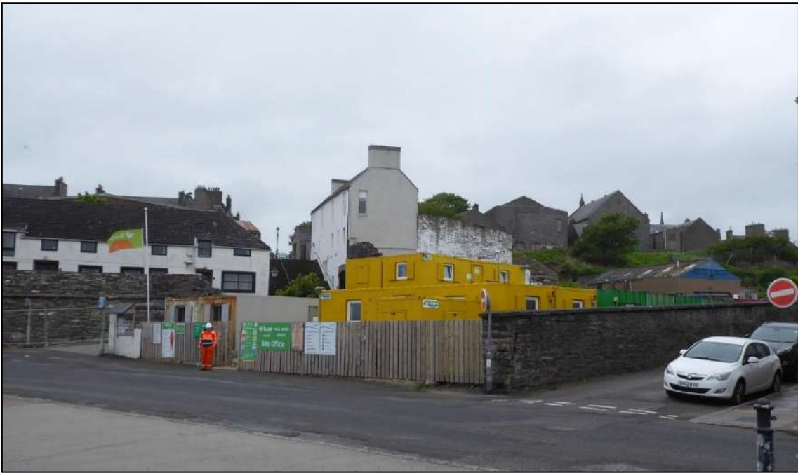
Figure 11: general view of the site in 2019 before the Beatrice construction site cabins were removed.
