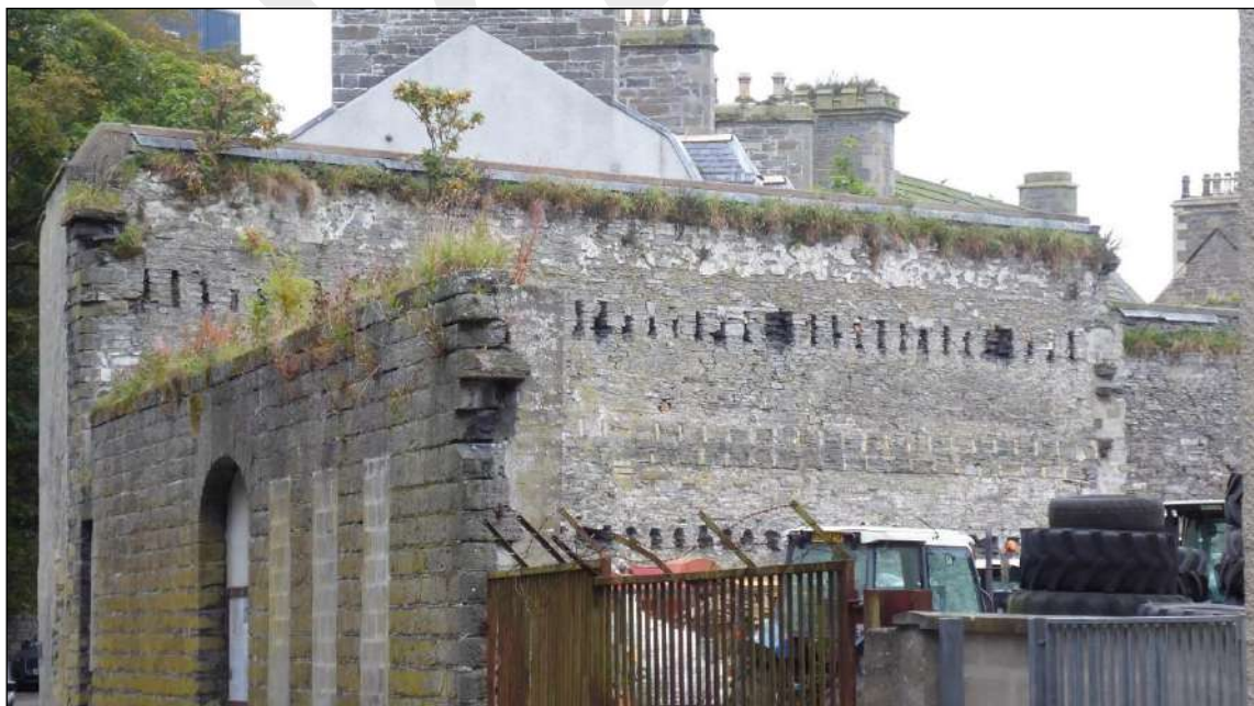
Figure 9: (top) part of the surviving elevation of the former Wick Steam Mills on Union Street with arched opening; (below) masonry side elevation also remaining.
