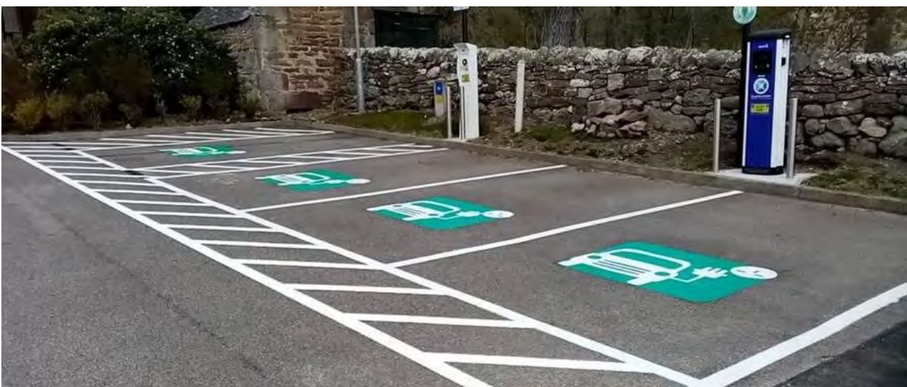
New electric vehicle charging points at Brora on the NC500.
