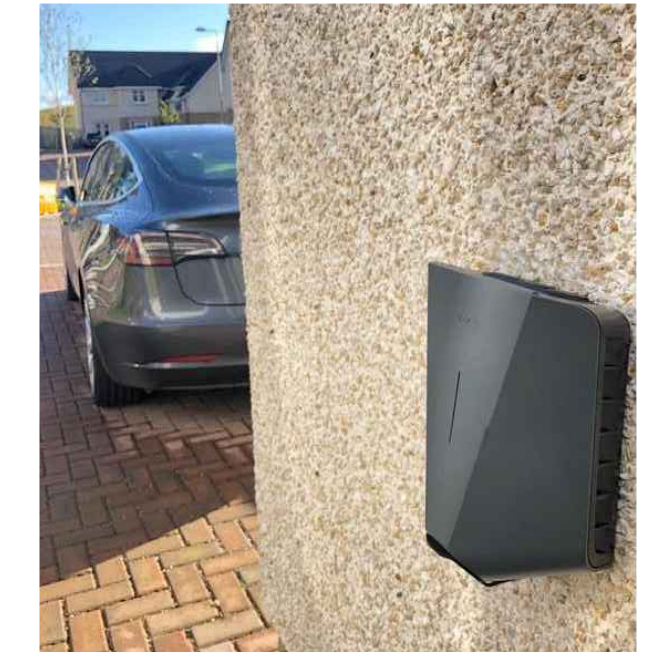
In-Curtilage charging provision
