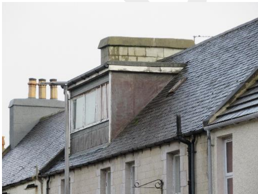
Example of unsympathetic box dormer
