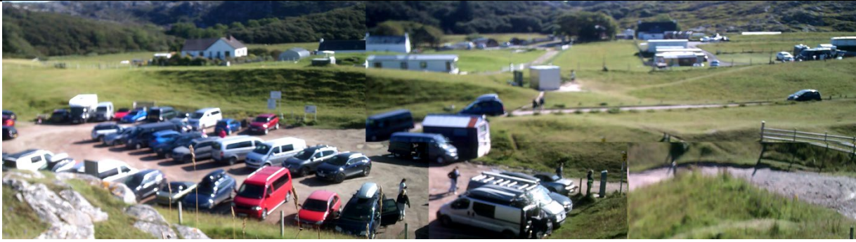
Images below show potholing of the car park surface between annual remedial works, from 2021:
