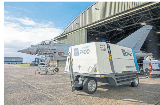
One of the new generators at RAF Lossiemouth.
