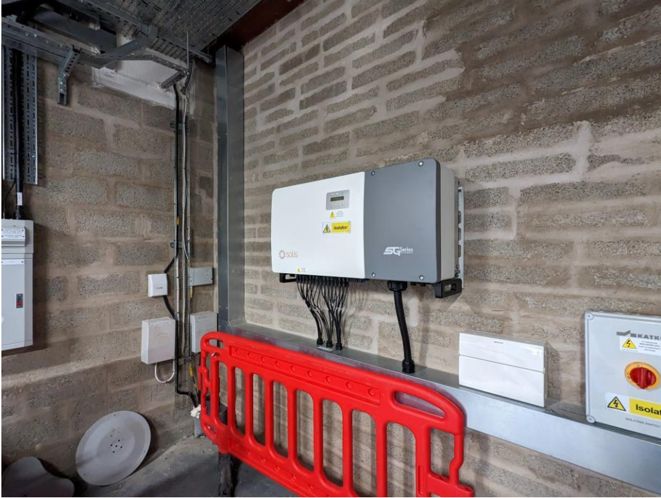
Figure 4-24: Highland Archive Solar Power panel
