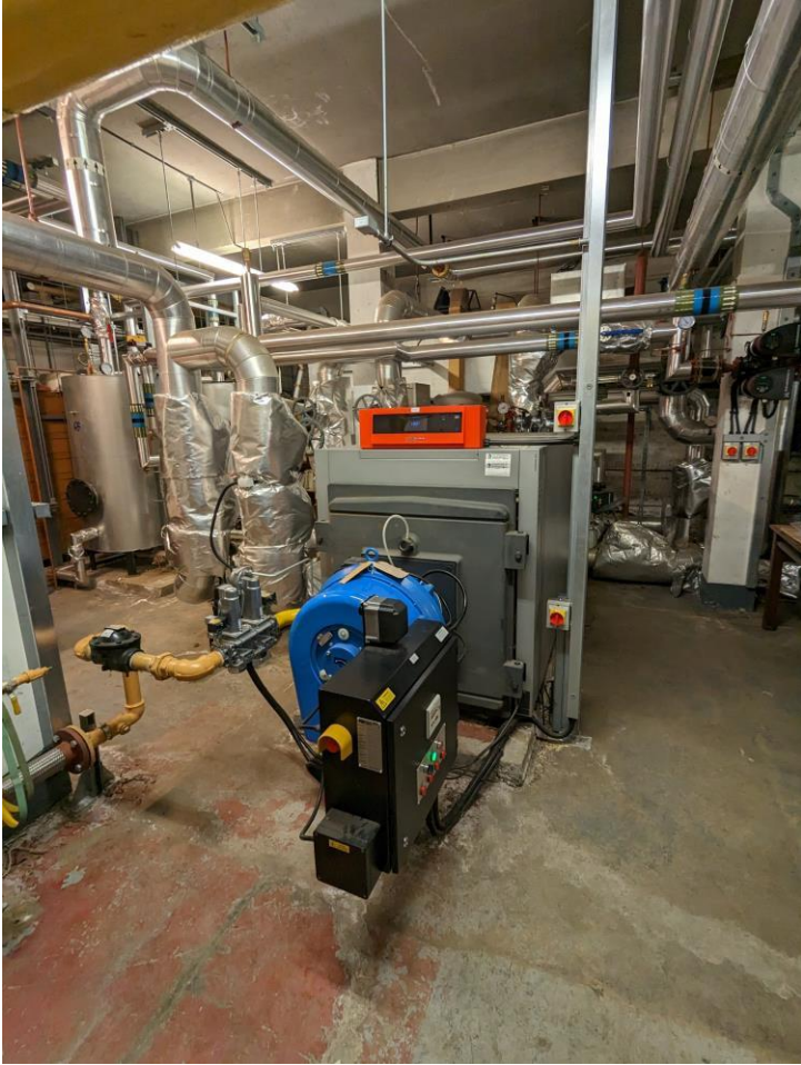
Figure 4-8: Highland HQ Gas Boiler
