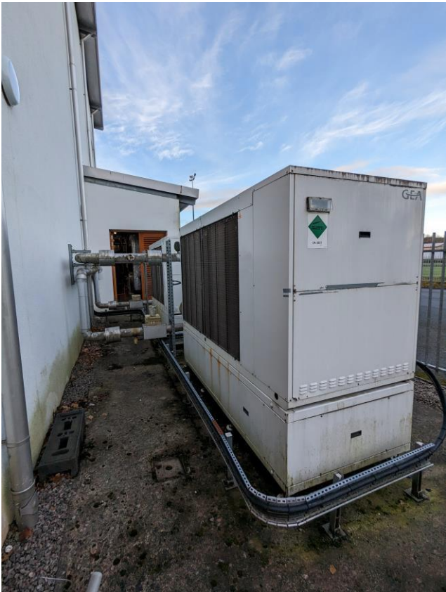
Figure 4-26: Highland Archive air-cooled chillers
