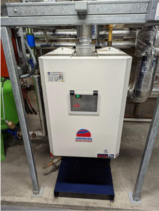
Figure 4-25: Highland Archive gas fired instantaneous hot water heater
