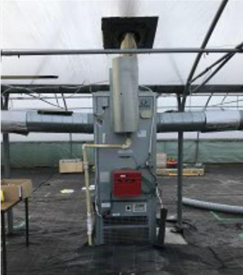
Figure 4-13 Polytunnel, kerosene boiler
