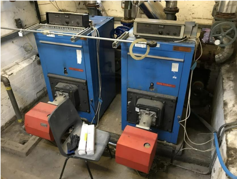
Figure 4-12 Existing gas-fired boilers, soon to be replaced with new gas-fired boilers
