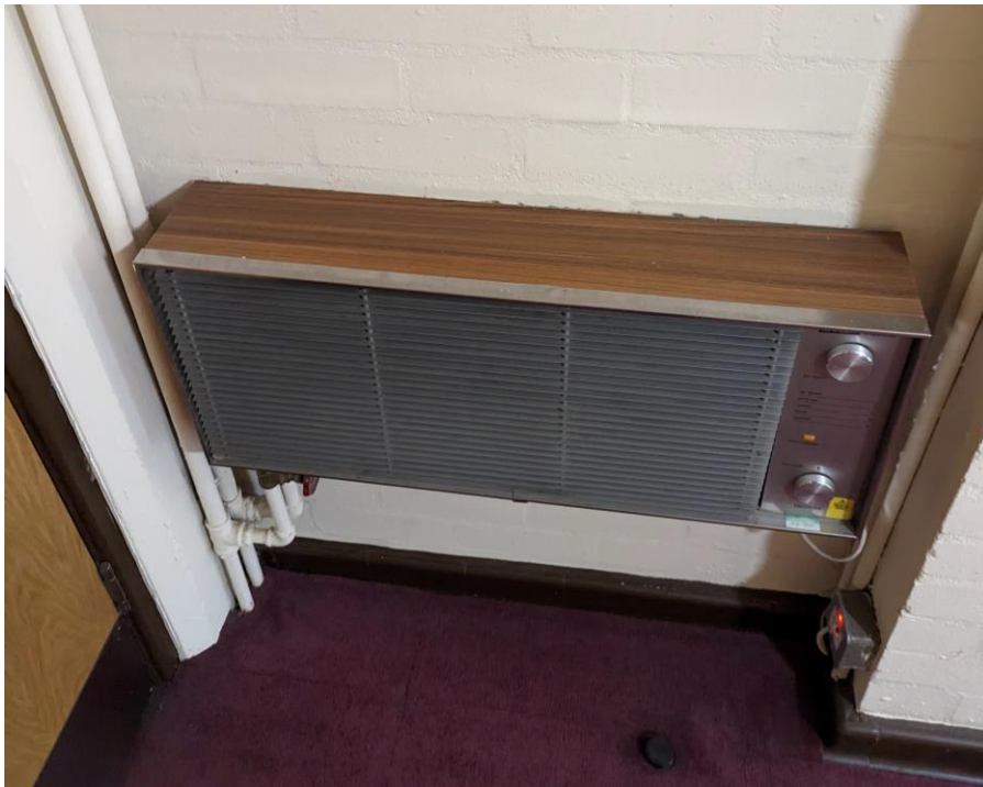
Figure 4-10: Highland HQ heater
