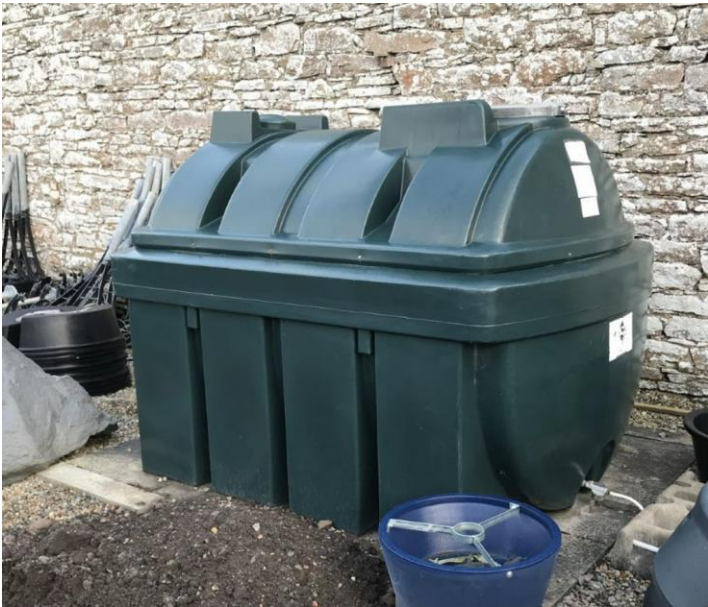
Figure 4-14 Kerosene fuel storage, at northern wall of site
