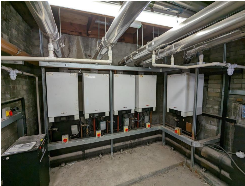
Figure 4.5: Inverness Town House Boiler Array
