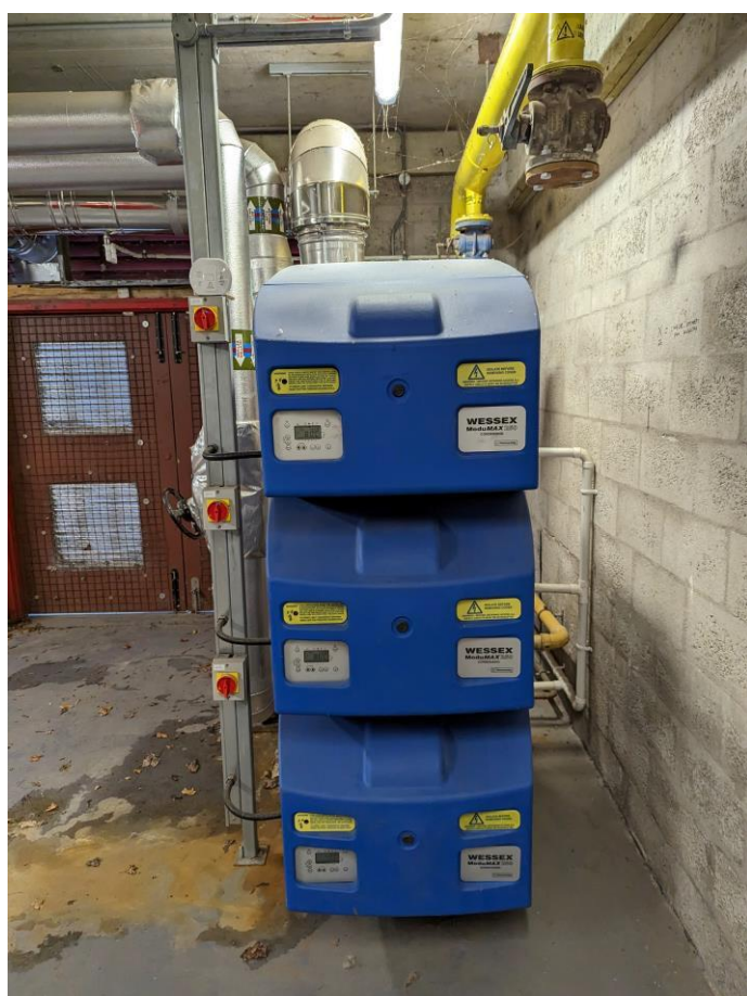
Figure 4-1: Leisure Centre dry-side gas boilers
