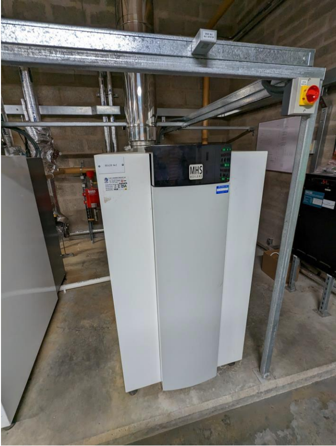
Figure 4-23: Highland Archive gas boiler
