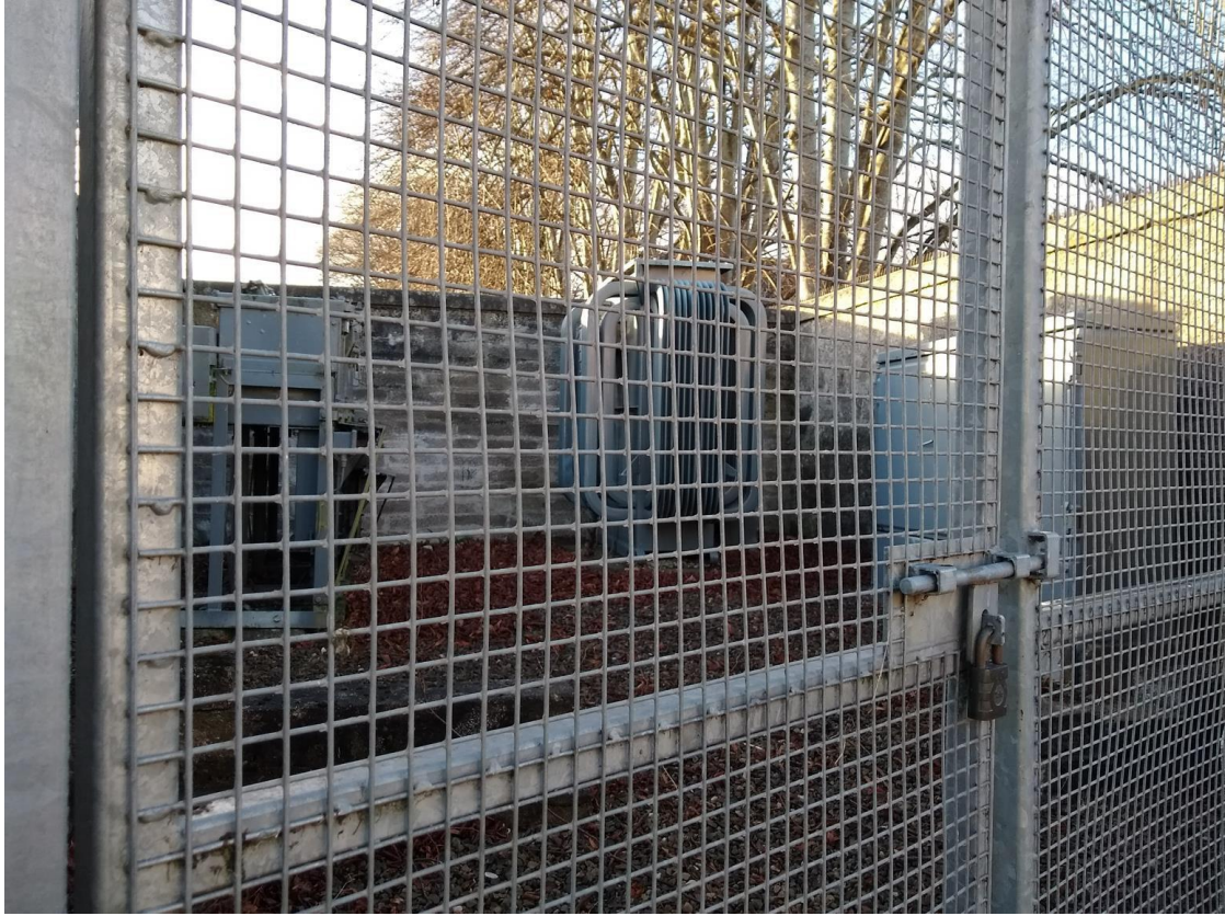
Figure 4-43 Existing substation on the north side of the Northern Meeting Park. An upgrade is planned for the electricity connection.
