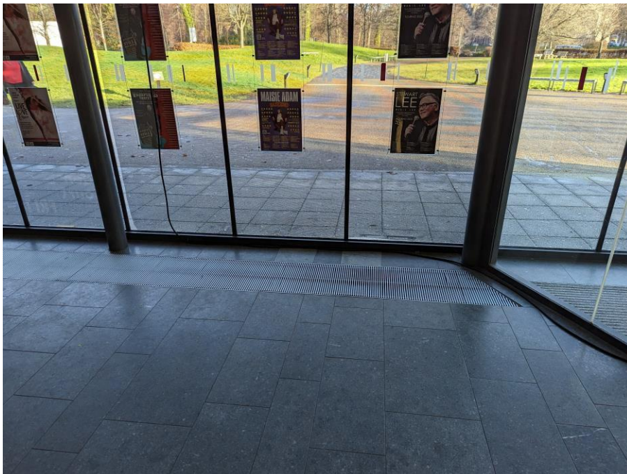
Figure 4-31: Trench heating near main entrance
