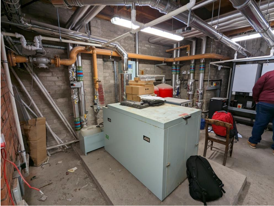
Figure 4.6: Inverness Town House CHP unit
