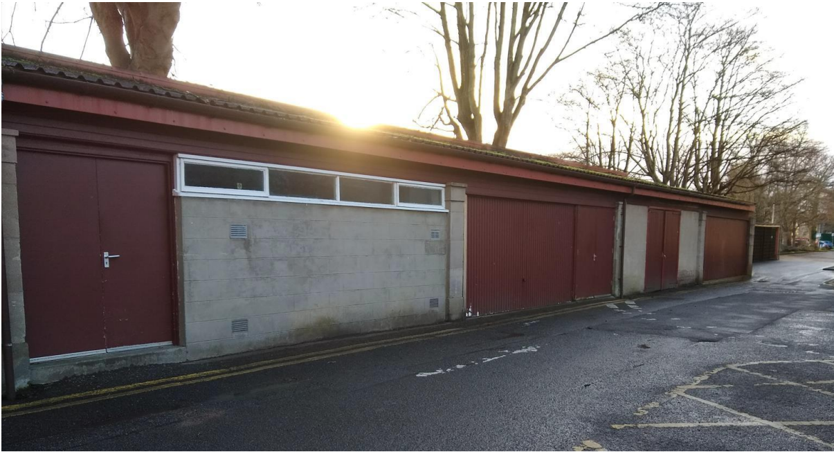
Figure 4-41 Storage structure, where an energy centre could be potentially located in the future. On Council HQ land, adjacent to the Northern Meeting Park, on the south side
