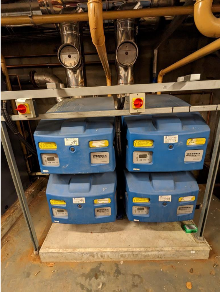
Figure 4-29: Main plantroom boiler plant
