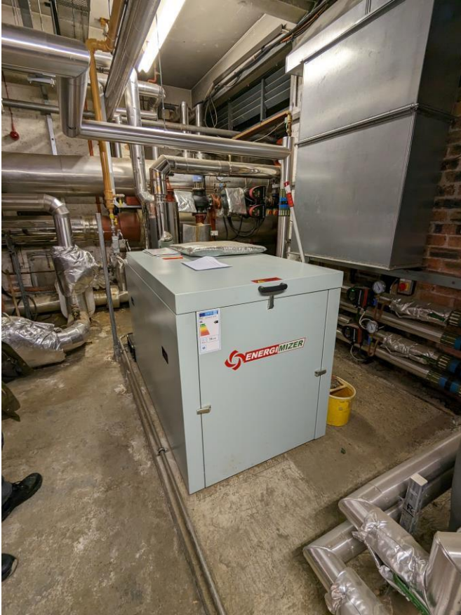
Figure 4-7: Highland HQ CHP Unit
