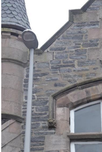
Historic movement on the front elevation is being monitored but will require repair.
