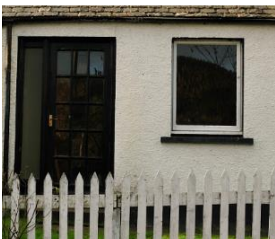
Fig. 68 Inappropriate replacement door and window
