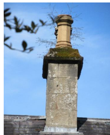
Fig. 55 Vegetation growing in chimney pots
