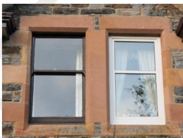
Fig. 69 Inappropriate replacement windows
