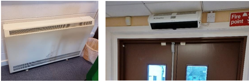
Figure 6: Small Classroom Heating (left); Corridor Over Door Heater (right)
