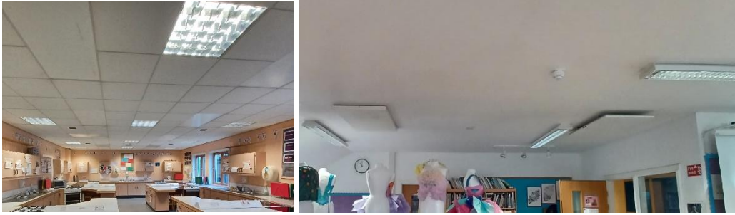
Figure 12: Typical Classroom Lighting – Ground Floor (left) and First Floor (right)
