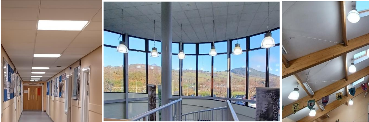
Figure 14: LED Lighting in Corridor (left), Library (middle) and Dining Hall (right)
