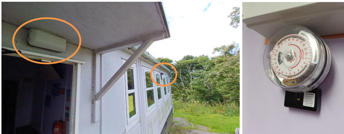
Figure 20: External security lighting (left); solar dial time switch control (right)
