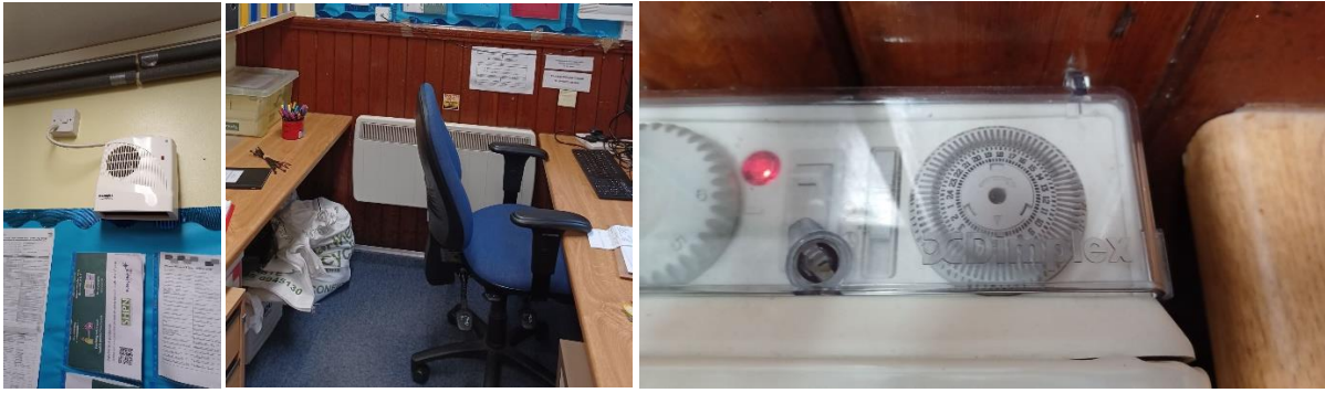
Figure 12: Office wall mounted element fan heater (left); convection heater (centre); convection heater controls (right)
