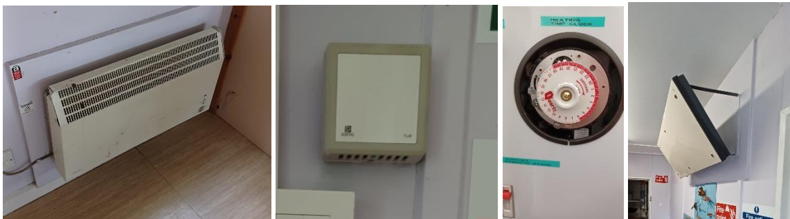
Figure 10: Canteen panel heater (left); Canteen thermostat (centre left); Heating timeclock control (centre right); Canteen Cloakroom wall radiant panel heater (right)
