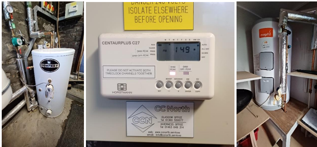
Figure 14: Main building hot water calorifier (left) and programmer control (centre); Canteen hot water calorifier (right)
