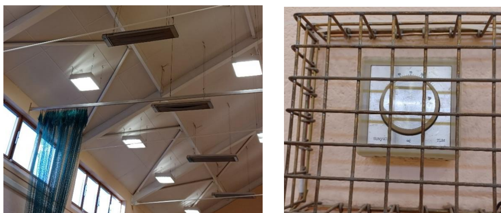
Figure 5: Games Hall Heating – heating units (left); thermostat control (right)
