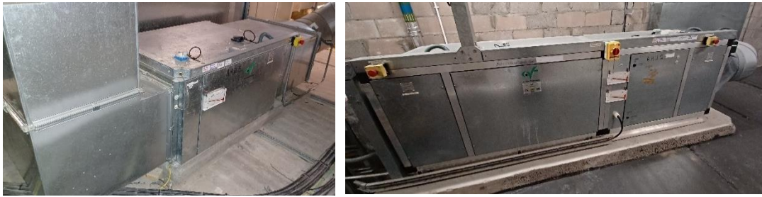
Figure 10: Changing Rooms (left) and Kitchen (right) Air Handling Units
