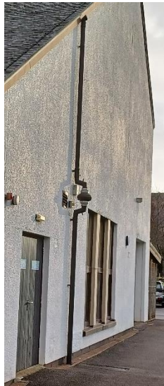
Figure 11: Radon Sump Pump Example
