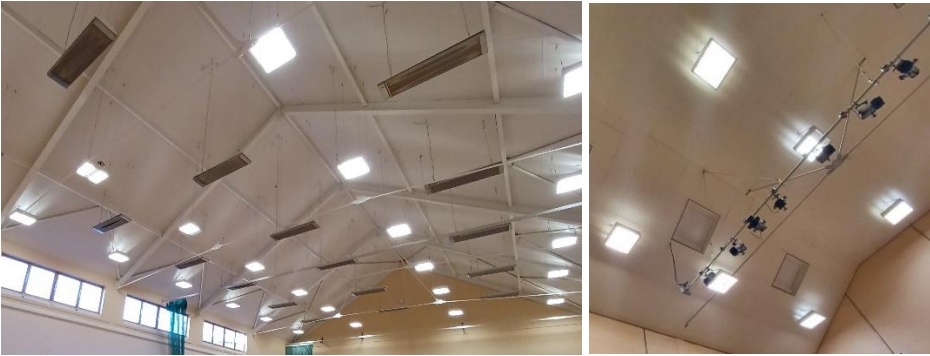
Figure 13: Games Hall (left) and Main Hall (right) Lighting
