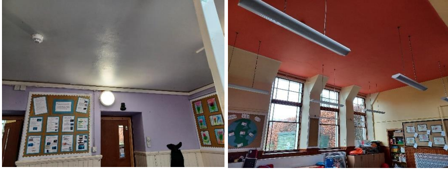
Figure 18: Typical LED lighting in school
