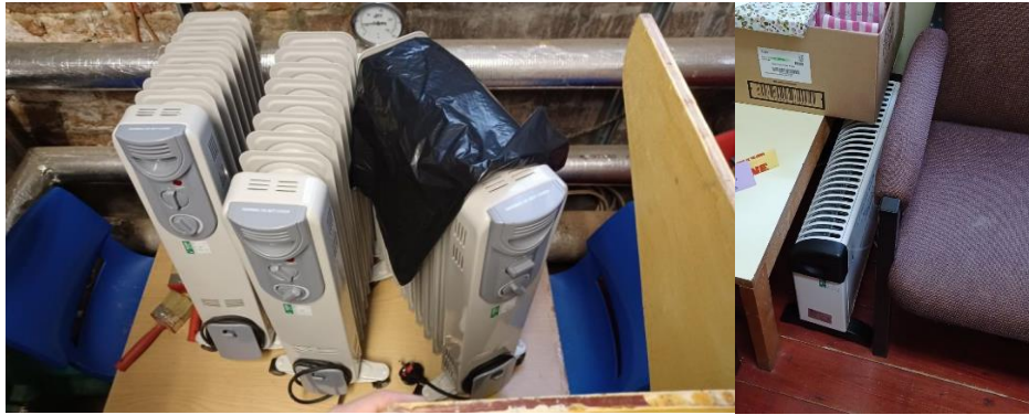
Figure 13: Portable heaters stored in Boiler Room
