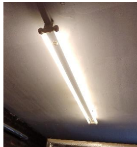
Figure 19: Ceiling mounted T8 fluorescent tubes with manual control in old Boiler Room
