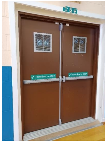
Figure 22: Games Hall Fire Doors (grilles for radon ventilation)
