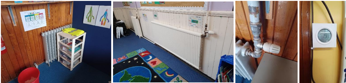
Figure 9: Typical heat emitters in Classroom (left) and Library & Circulation Space (centre left); Typical controls on radiators in Classrooms, Library and Circulation Space (centre right); room thermostat in Classroom (right)
