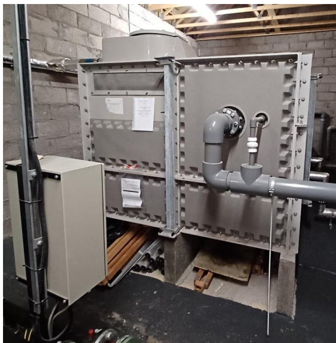
Figure 9: Cold Water Storage Tank
