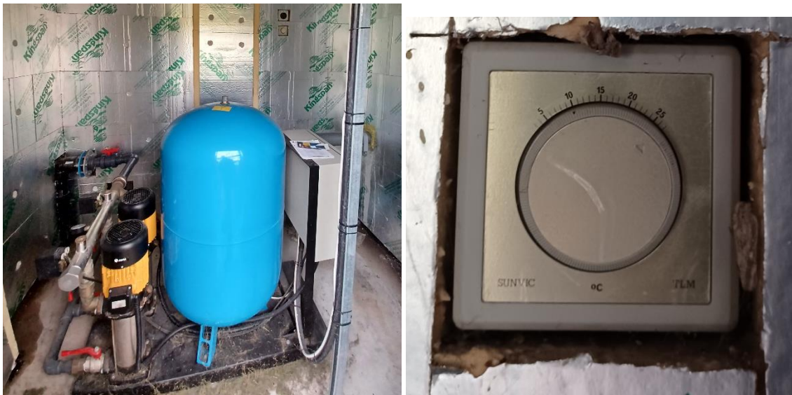
Figure 23: Inside Pump House (left) Pump House Thermostat 26°C (right)
