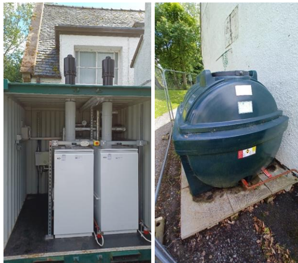
Figure 8: Two temporary oil boilers (left); 2,500l oil tank (right)
