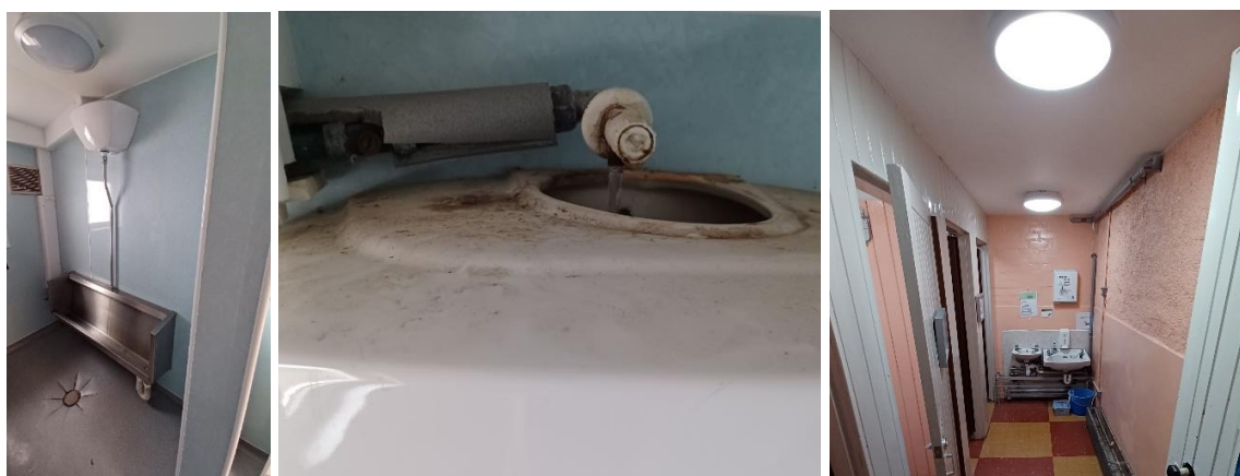
Figure 15: Urinal (left) and controls (centre); Dripping tap in Girls WC (right)
