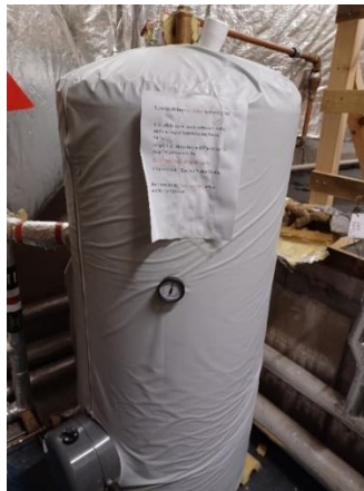
Figure 7: Kitchen hot Water calorifier
