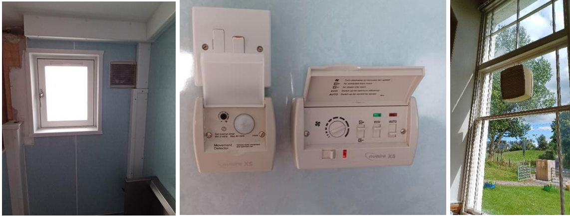
Figure 16: Wall mounted extract fans in WCs (centre left); Extract fan controls in boys WC (centre right); Extract in Classroom (right)
