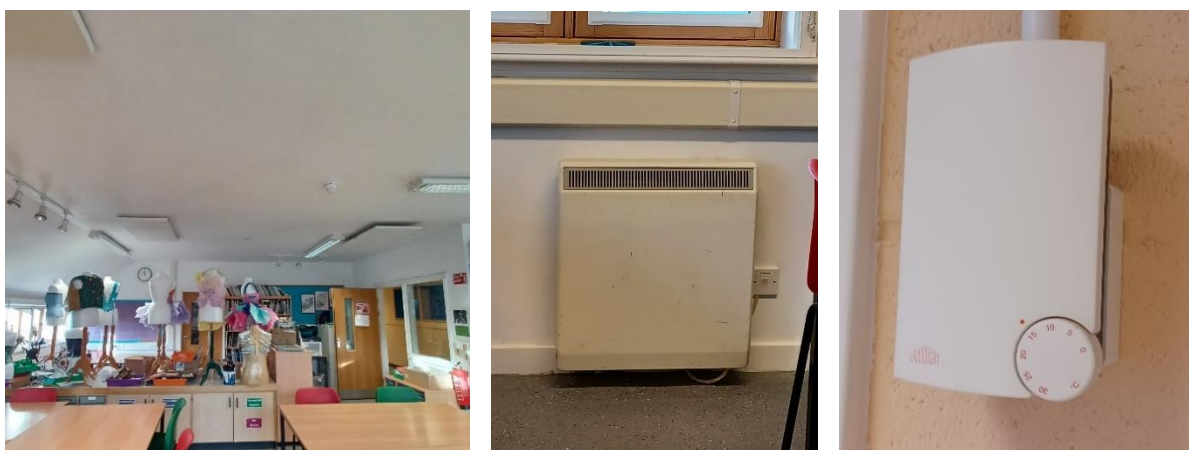
Figure 4: Typical Classroom Heating – ceiling-mounted electric radiant panel heater (left); electric storage heaters (middle); controls for panel heaters (right)
