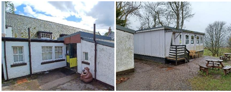
Figure 3: Broken fascia board (left); moss and lichen on roofs and walls (left and right); moss in gutter (right)
