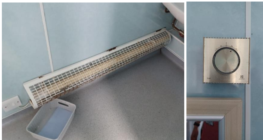
Figure 11: Electric tube heaters in WCs (left); thermostat controls in WCs (right)
