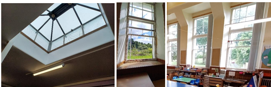
Figure 2: Single glazed rooflight with cracked panes (left); single glazed windows with rotten/flaky paint frames (centre); blinds removed from south-facing double height windows (right)
