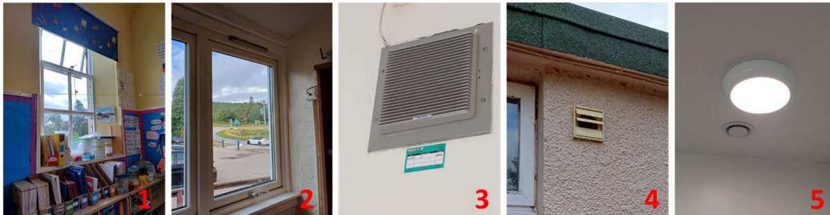
Figure 16: Openable DG windows (no tricklevents) [1]; Openable DG windows (tricklevents) [2]; Extract in Kitchen [3]; Vent (North Block WCs) [4]; MV System Outlet (Nursery) [5]
