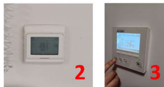
Figure 18: Air Source Heat Pump System (External Unit [1]; Room Thermostat [2]; Programmer [3])
