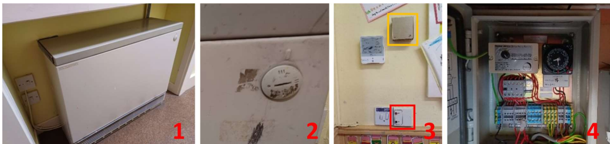
Figure 13: Storage heater [1]; Dial Controls [2]; Room Thermostat (yellow box) and Boost Control (red box) [3]; Weather Watcher Control [4]
