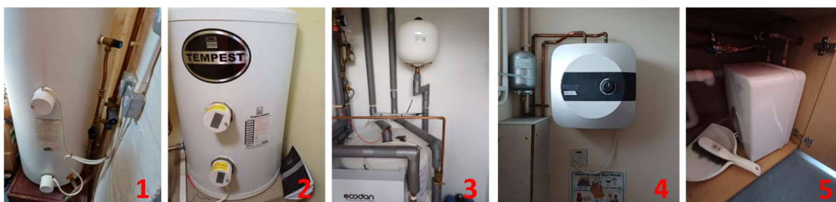
Figure 15: Electric Immersion Calorifier (Horsa Hut) [1]; Electric Immersion Calorifier (South Block WCs) [2]; Hot Water Calorifier (Nursery) [3]; Point-of-Use Water Heater (North Block WCs) [4]; Under sink Point-of-Use Water Heater (Cloak/Craft Area) [5]
