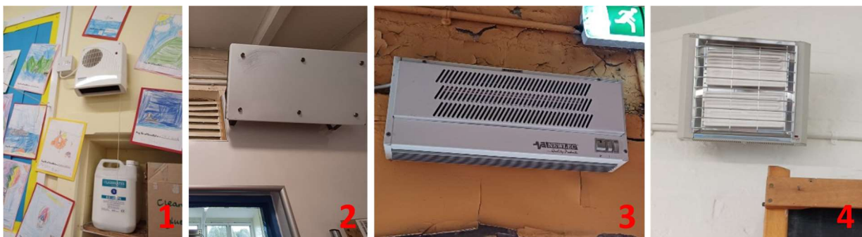
Figure 14: Wall Fan Heater (Classroom) [1]; Radiant Panel Heater (Kitchen Store & Cleaner's Cupbd) [2]; Overhead Air Heater (Horsa Hut) [3]; Infrared Heater (Horsa Hut) [4]
