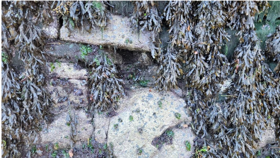
Photo 24: Voids in Wall at Rock Masonry Interface
