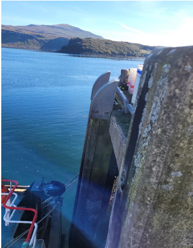
Photo 14: Pier Fenders with Steel Caps
