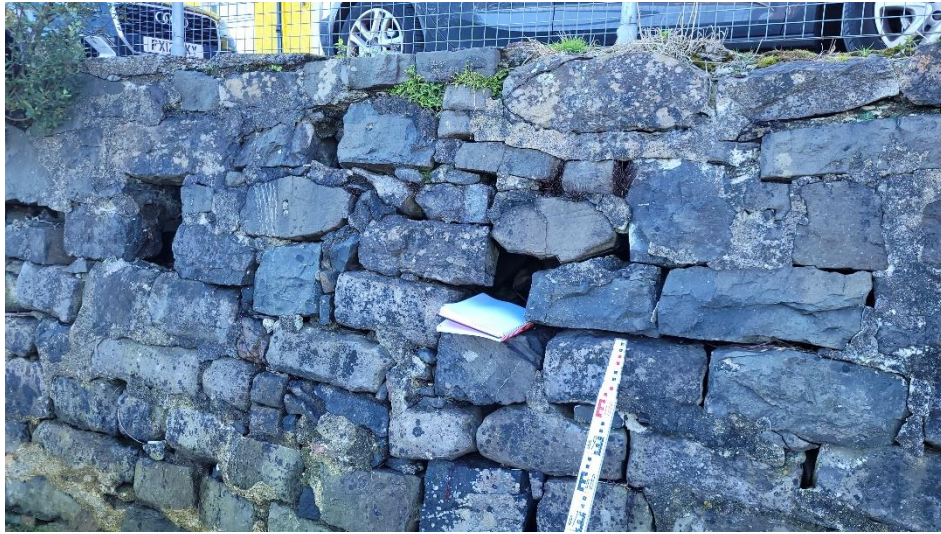
Photo 20: Missing Stones in Retaining Wall above Slipway
