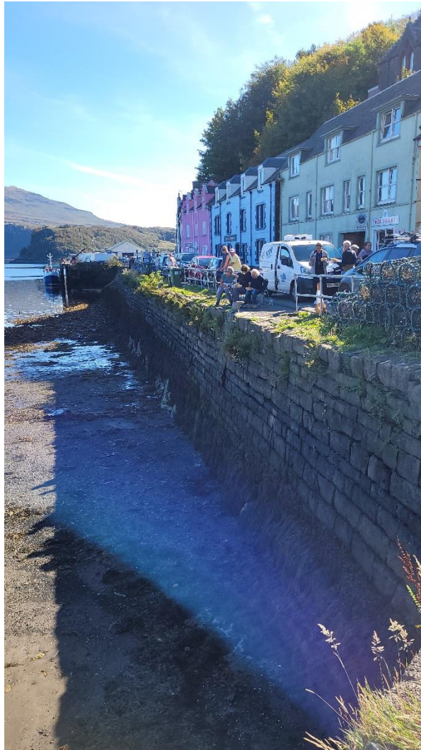
Photo 22: Missing Handrailing along Quay Street
