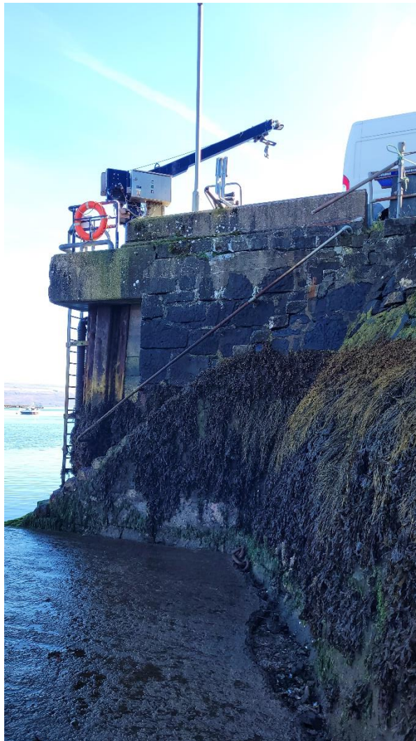
Photo 21: Eroded Channel at Back of Slipway
