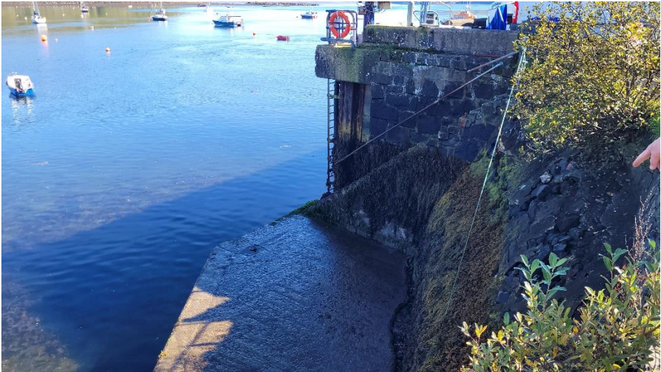
Photo 19: Bulge in Wall
