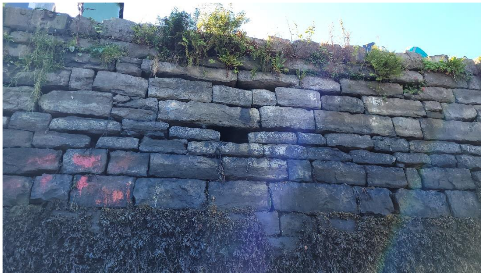
Photo 23: Open Joints & Missing Stones at Quay Street Retaining Wall
