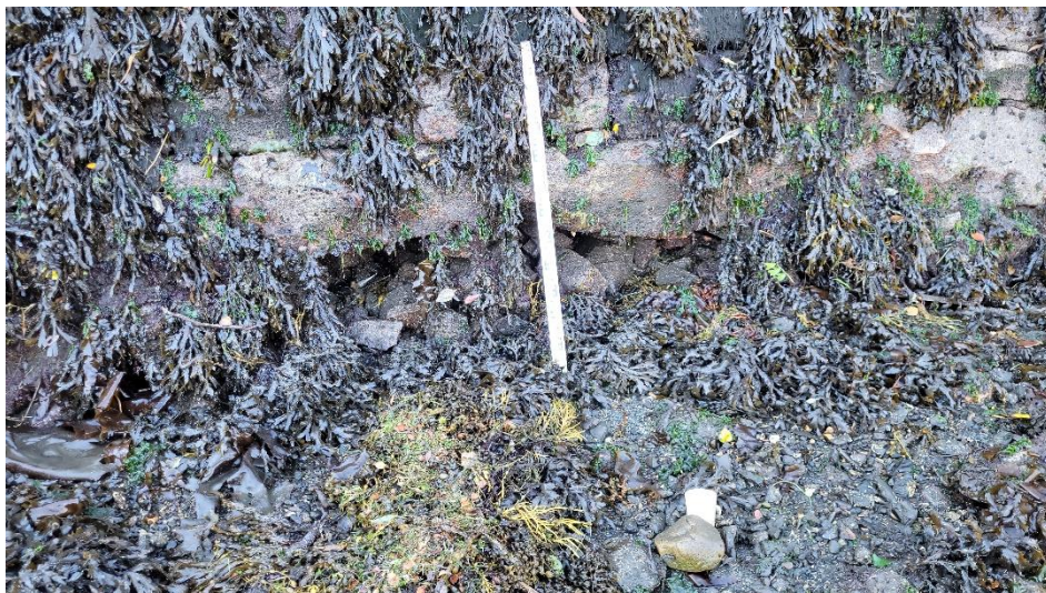
Photo 26: Undermining of Masonry Wall
