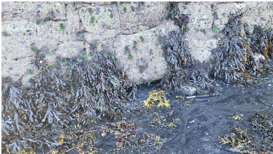
Photo 25: Undermining of Masonry Wall
